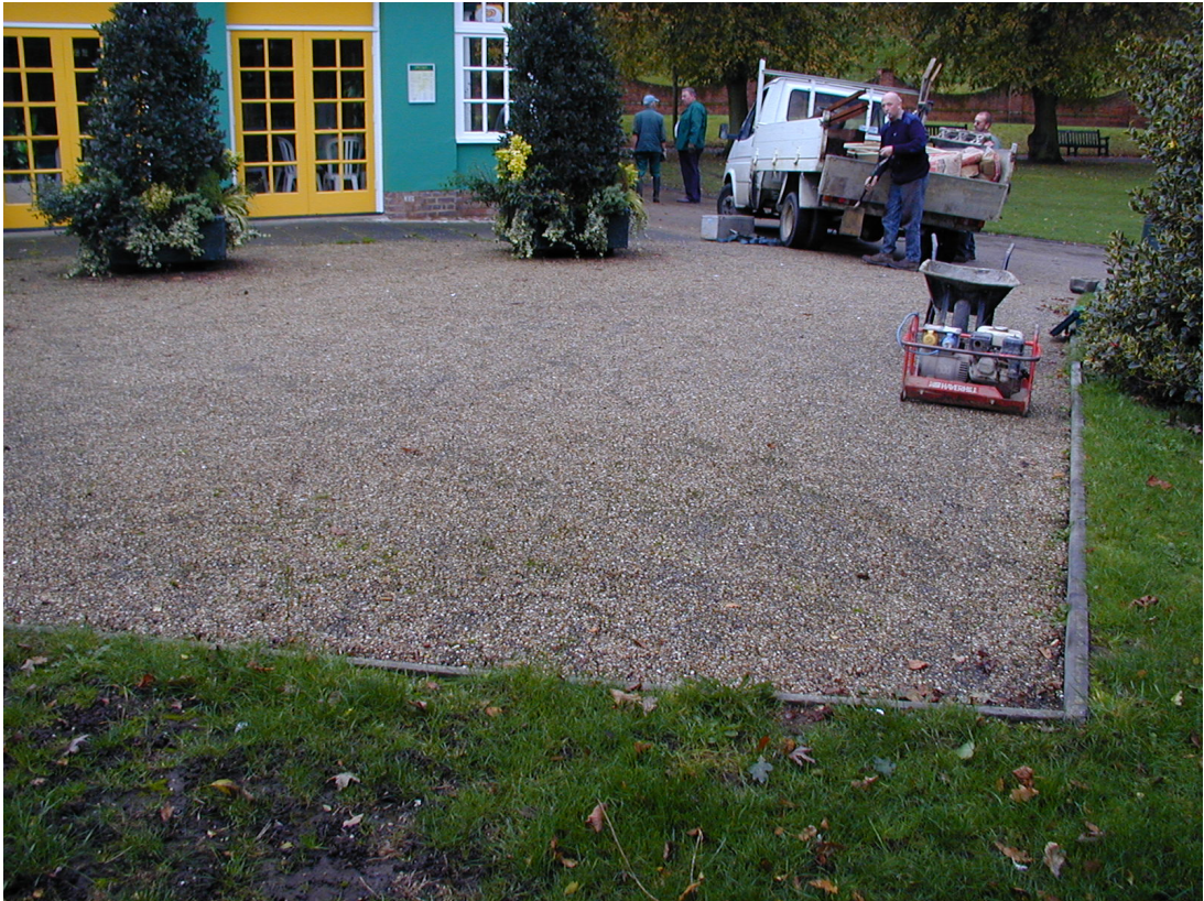
Fig 1 Photograph before work on the base of the telephone box, looking south-west.
