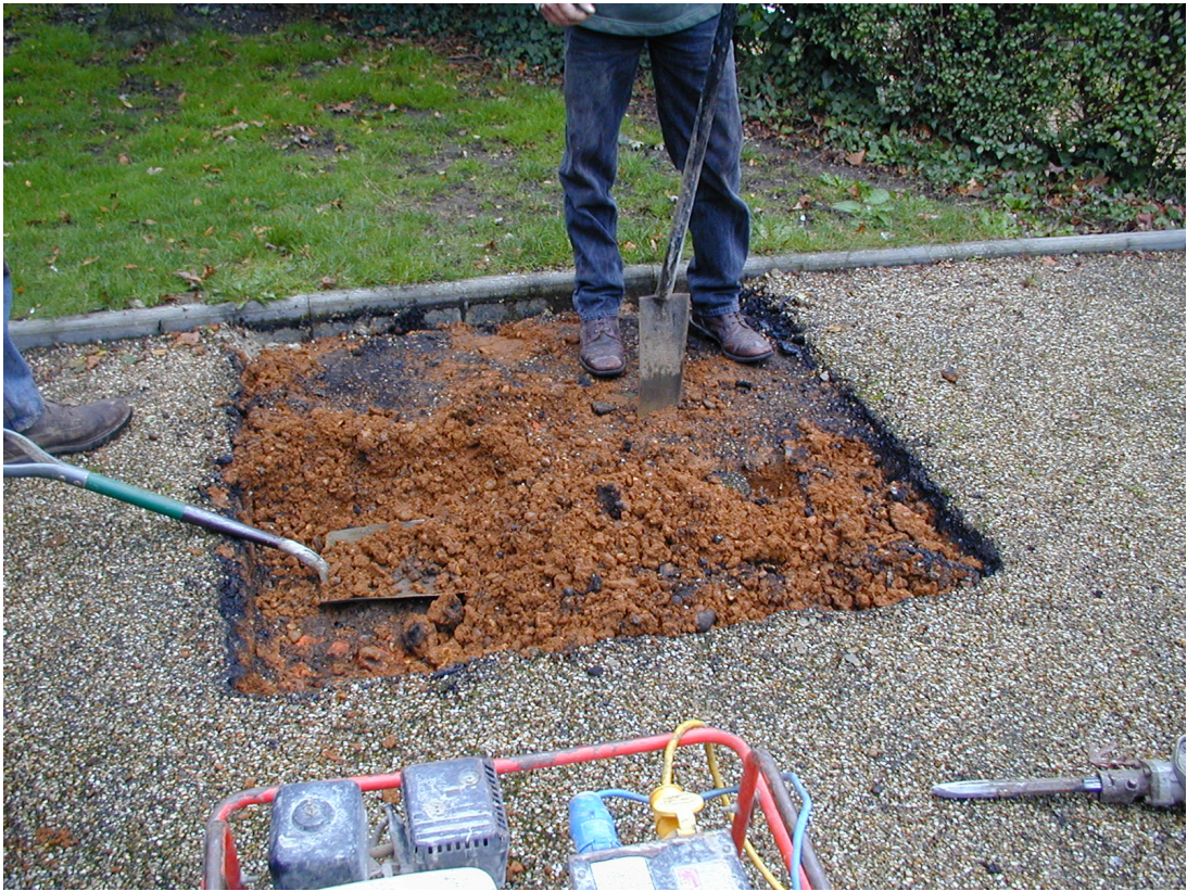
Fig 2 Photograph during work on the base of the telephone box, looking north-east.
