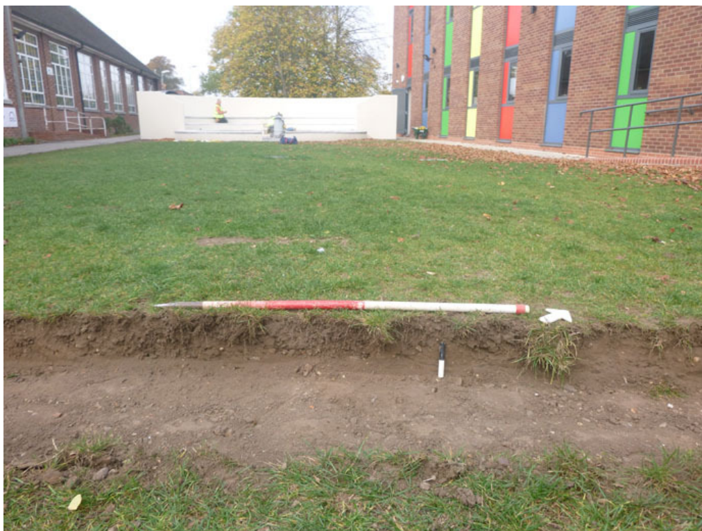
Photograph 9 Excavation depth for slabs of 100mm, dug through modern topsoil, looking W
