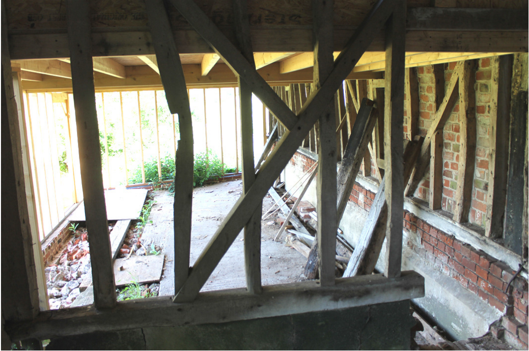
Photograph 17 Western elevation of midstre, showing y-bracing and modern hole for access into Building C. Photograph taken facing west.
