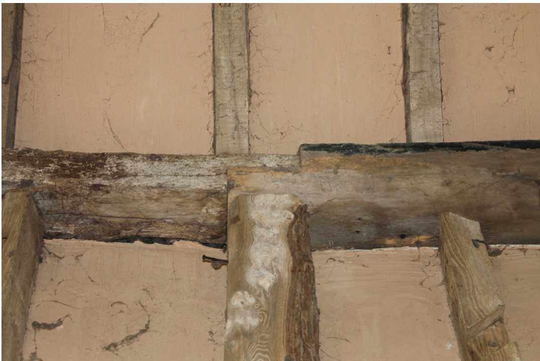
Photograph 20 Modern timber (right) jointed with original wall-plate (left) in bay 3. Modern hand-sawn supporting post visible. Photograph taken facing north.
