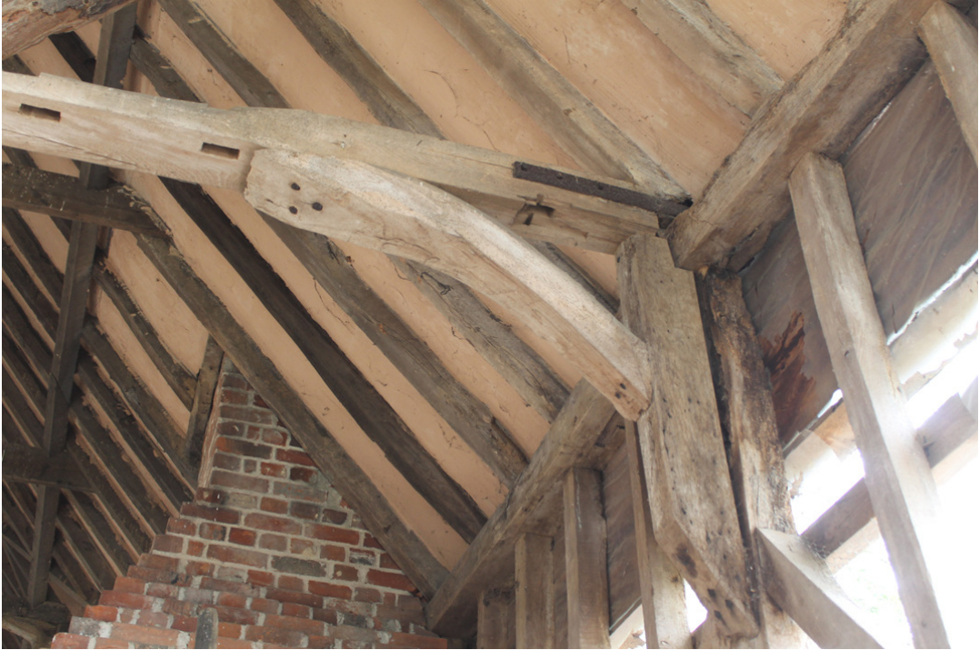
Photograph 11 Southern end of tie beam between Bays 1 and 2, with additional pieces of timber and modern hand-sawn arch brace. Photograph taken facing east.
