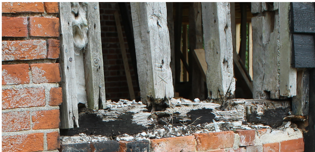
Photograph 21 Carpenter's mark visible on exterior of stud in western elevation of Bay 1. Photograph taken facing south-east.
