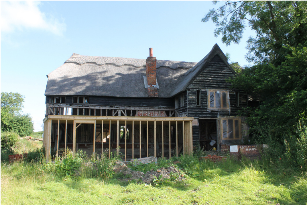
Photograph 1 South elevation of barn, with modern building on footprint of Building C in foreground – photograph taken facing north.
