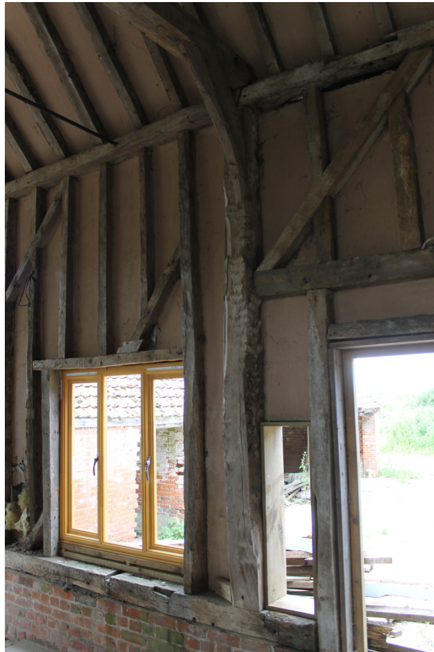
Photograph 16 Modern hand-sawn timber forming northern principal post supporting the tie beam between Bays 2 and 3. Photograph taken facing north-west.
