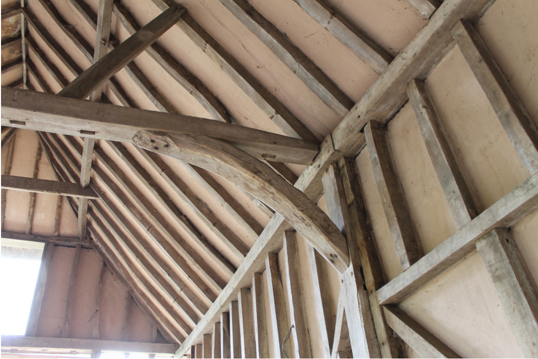
Photograph 15 Northern end of tie beam between Bays 1 and 2. Shows re-used tie beam and modern hand-sawn arch brace. Also visible is the joint between the wall-plates. Photograph taken facing north-west.
