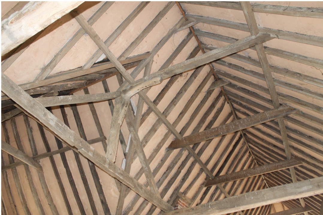
Photograph 14 Shot of bracing arrangement of timbers at intersection of midstrey and main range. Photograph taken facing south-west.
