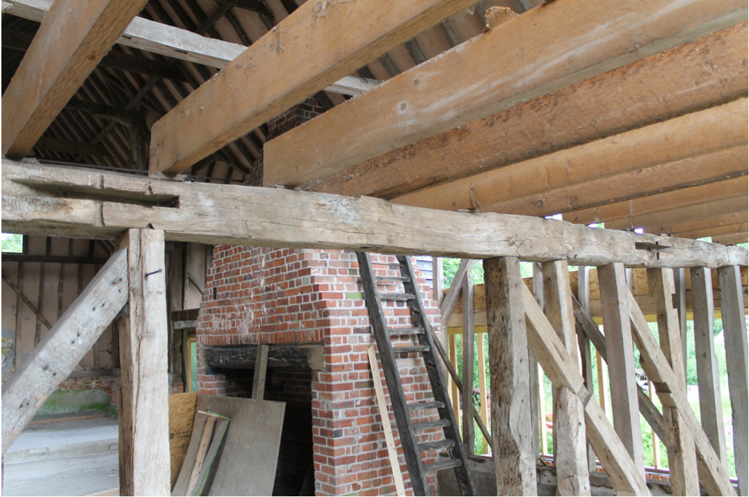
Photograph 9 Back of the beam supporting the inserted floor in Bay 1, showing disused mortices in the old timbers. Photograph taken facing south-east.
