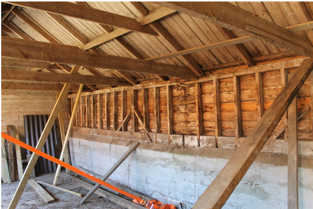
Photograph 6 Interior of Building B, showing original machine cut timber on eastern elevation – photograph taken facing north-east.
