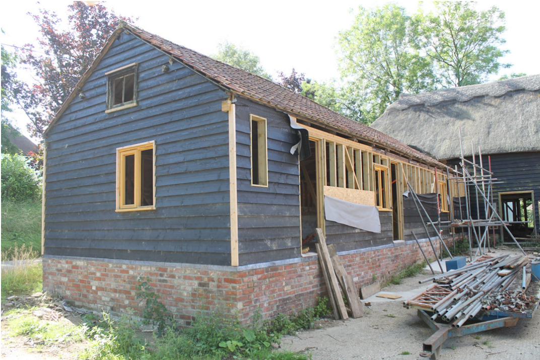
Photograph 5 West elevation of Building B, with multiple modern timbers visible – photograph taken facing south-east.
