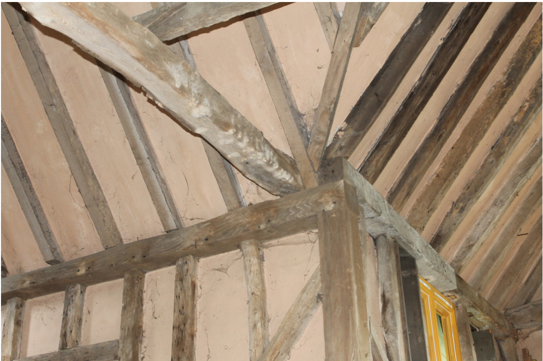
Photograph 12 Modern hand-sawn tie beam between Bays 3 and 4, on the southern elevation. Also visible is the midstrey and modern wall plate joining the original. Photograph taken facing south-east.
