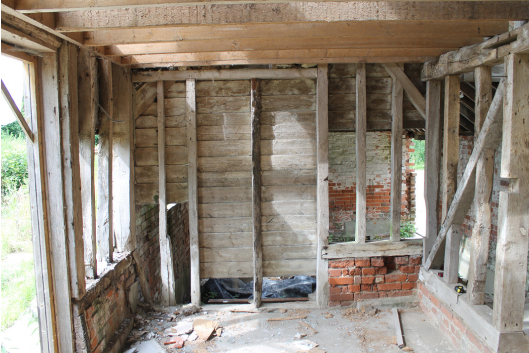
Photograph 19 Blocked ?original entrance into barn on northern elevation of bay 1. Photograph taken facing north.
