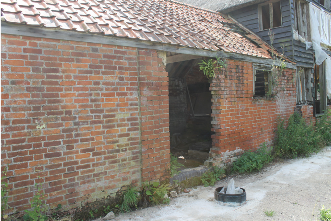
Photograph 3 West elevation of Building A, showing clear change in brickwork between two phases of construction – photograph taken facing south-east.
