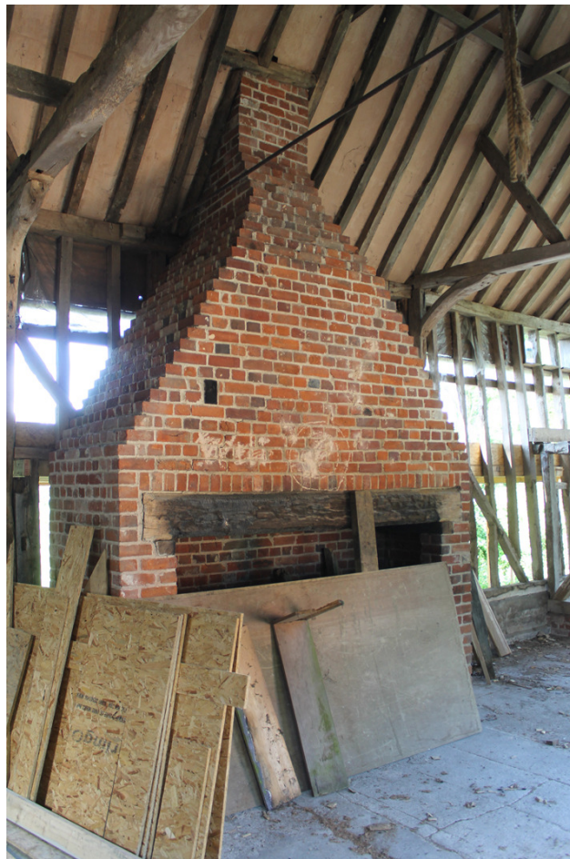
Photograph 10 Inserted modern brick oven in south of Bay 2. Photograph taken facing south-west.
