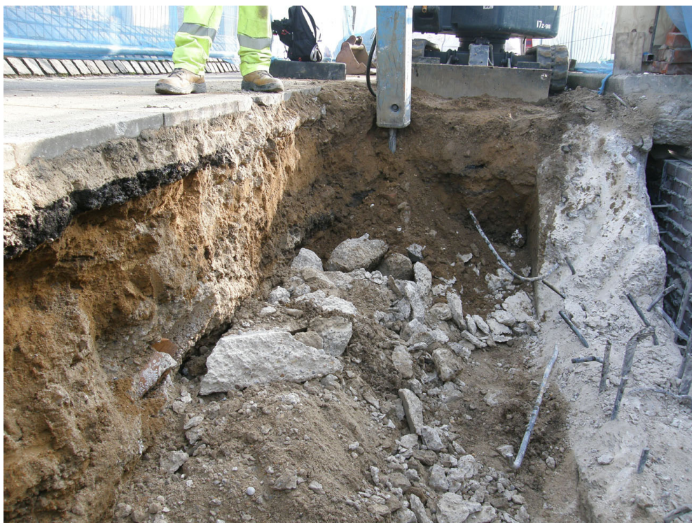
Photograph 2 Trench on east side of footbridge showing concrete abutment wall and made-ground, looking S
