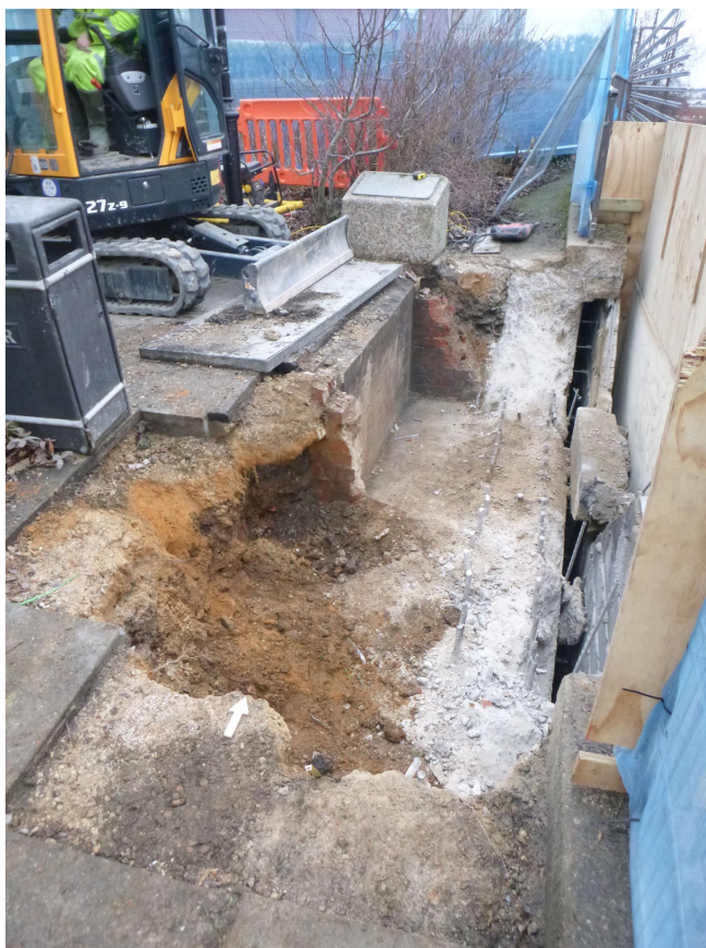
Photograph 1 Trench on west side of footbridge, the concrete abutment wall, brick inspection pit and made-ground can be clearly seen, looking N
