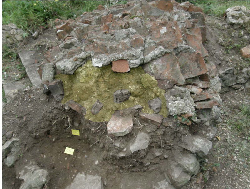
Photograph 2 Detail of collapsed masonry after cleaning. Original Roman mortar highlighted in section. Photograph taken facing south-west.
