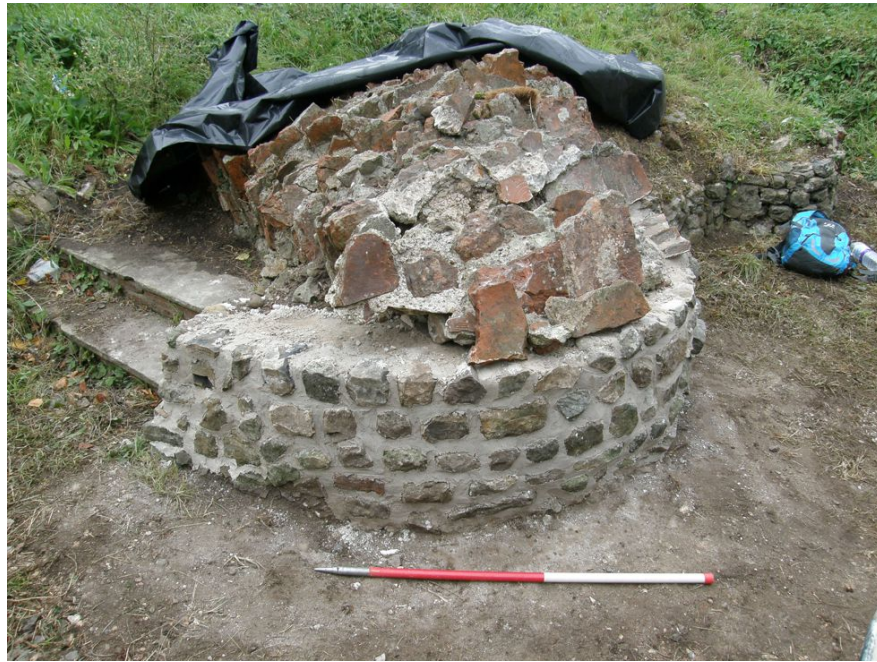
Photograph 4 Masonry during conservation work, showing partial reattachment of tile courses. Photograph taken facing south-west.
