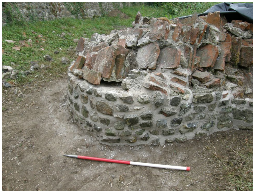
Photograph 5 Masonry during conservation work, showing partial reattachment of tile courses. Photograph taken facing south-east.
