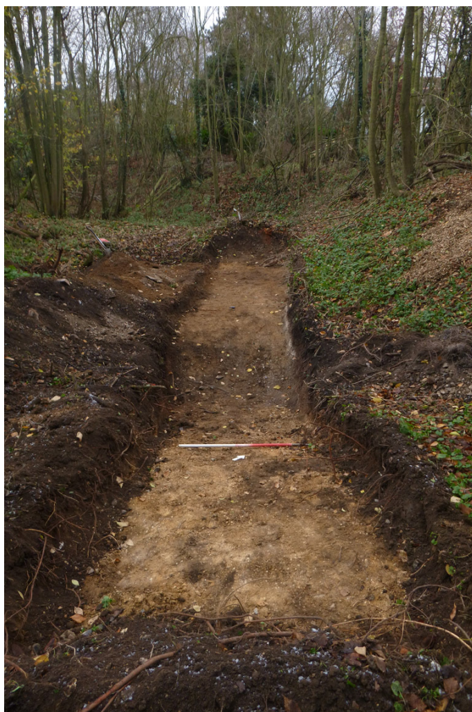
Photograph 4 T5, showing difference in ground level in the southeastern corner, looking NW
