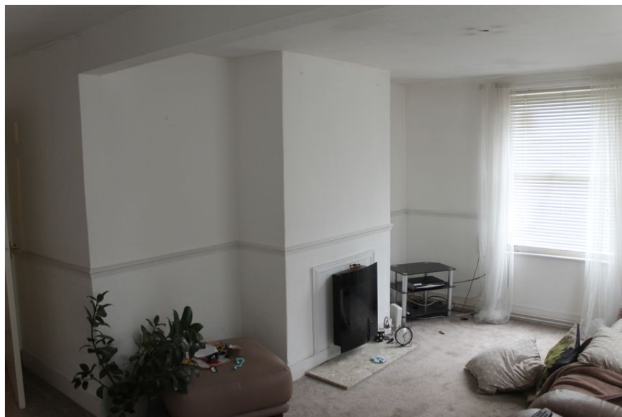
Photograph 22 Blocked fireplace in living room in first-floor of pub (replaced with electric heater). Photograph taken facing north.
