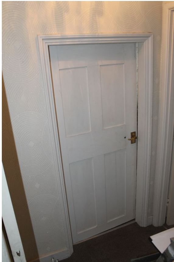
Photograph 21 Original four-panel door leading into northern bedroom on first-floor of pub. Photograph taken facing north-east.
