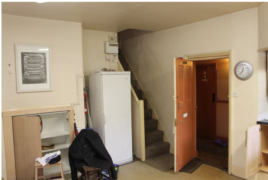
Photograph 20 Interior ground-floor of extension A, showing the blocked fireplace, door into corridor and stairway to first-floor. Photograph taken facing south.
