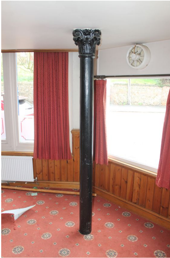
Photograph 19 Metal post in northern bar, supporting the first-floor. Note ornate decoration at apex. Photograph taken facing north-east.
