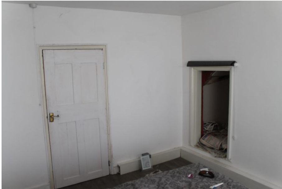
Photograph 23 Interior of northern bedroom in pub, showing original door (to left) and crawl-space into loft of extension A (to right).
