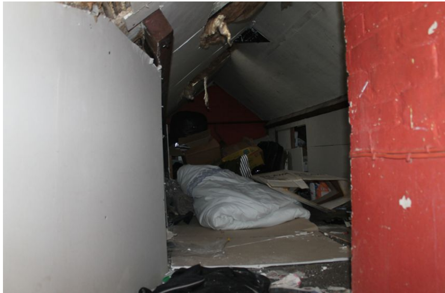
Photograph 24 Loft above extension A. Lath and plaster visible behind panelling. Chimney-stack visible to right. Photograph taken facing north-west.
