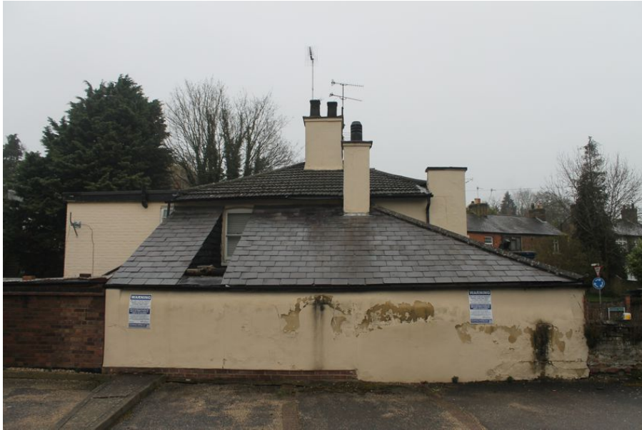
Photograph 6 Exterior of Bricklayers Arms showing extension B in foreground. Photograph taken facing north-east.
