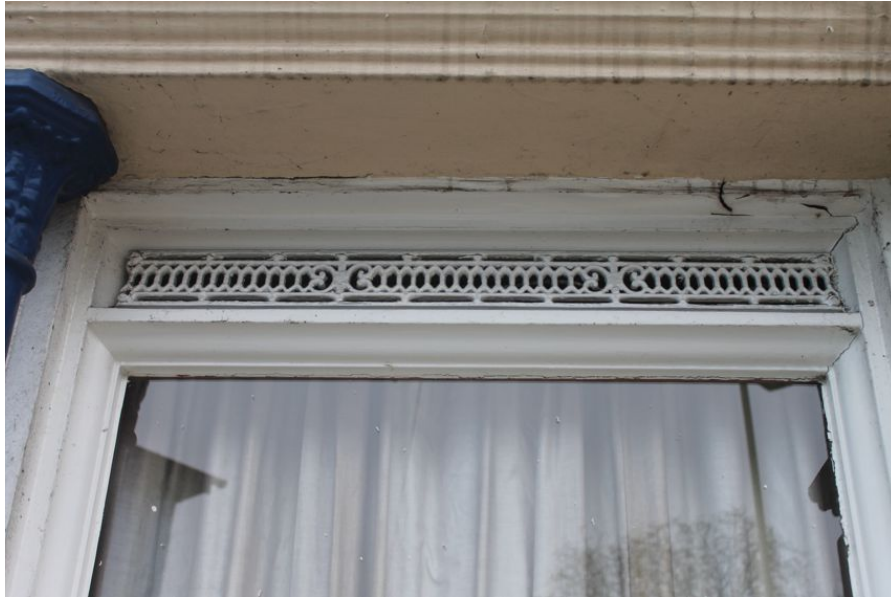
Photograph 10 Detail of vents above fixed windows on south-east elevation. Photograph taken facing north-west.
