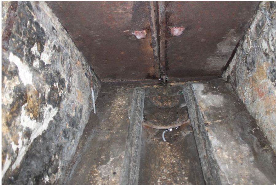
Photograph 12 Interior of cellar, showing hatch onto pavement and chute into cellar. Photograph taken facing north-west.
