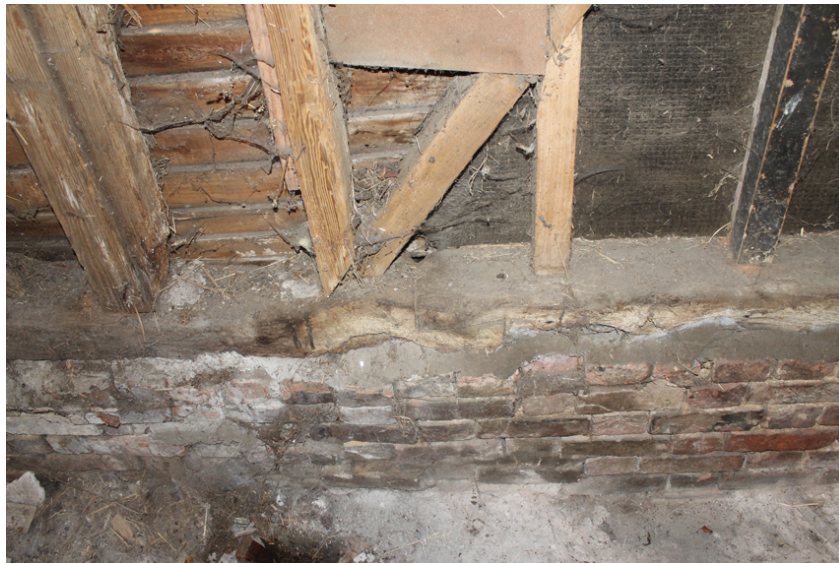
Photograph 18 Scarf joint on southern sill-beam in bay 3. Edge-halved scarf with square abutments. Photograph taken facing south.
