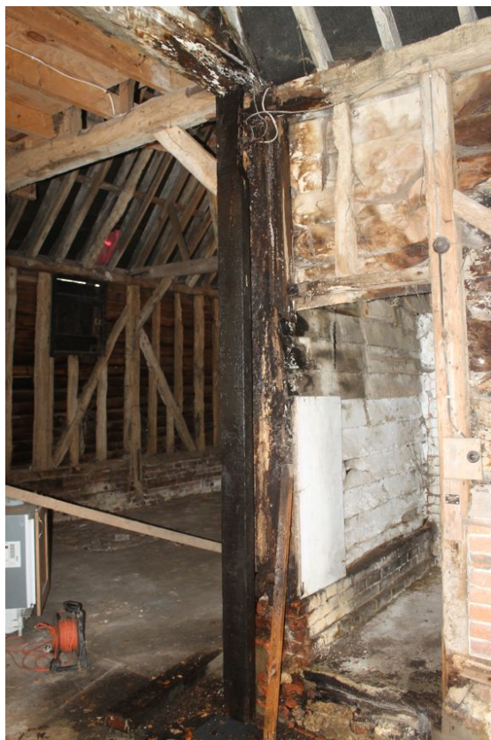
Photograph 11 The heavily water-damaged eastern principal-post between bays 2, 3 and the midstrey. Photograph taken facing north-west.
