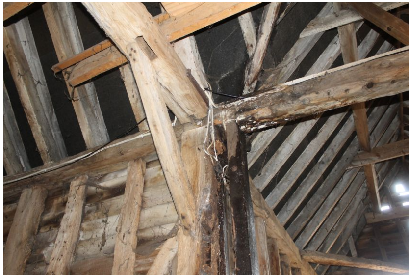
Photograph 22 Apex of principal-post on eastern elevation between bays 2 and 3. Showing heavy water-damage, empty mortise on tie-beam and scarf joint to immediate south (right) of principal-post. Photograph taken facing north-east.
