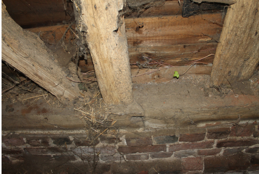
Photograph 17 Scarf joint in sill-beam on western elevation of bay 1. Appears to be rotated 90 degrees. Photograph taken facing west.
