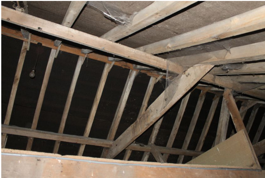
Photograph 2 Interior of Building A, showing roof truss and timbers. Photograph taken facing south-west.
