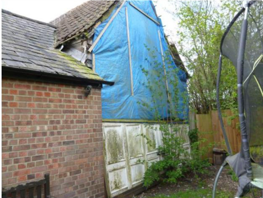
Photograph 6 North elevation of barn, covered in a tarpaulin. Photograph taken facing south-west. Taken from Planning Statement (2016).
