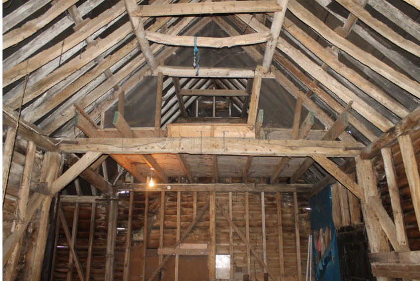
Photograph 15 Truss between bays 2 and 3. Also visible is the inserted attic floor above bay 3. Photograph taken facing south.
