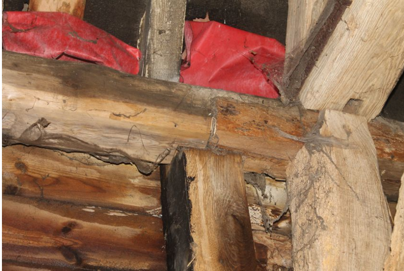
Photograph 21 Scarf joint immediately to south of principal-post between bays 2 and 3, on western elevation. Also visible are Baltic shipping marks on the end of the southern timber (the leftmost). Photograph taken facing west.
