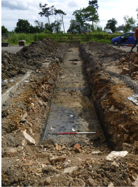
Photograph 5 Long shot of T2, showing unexcavated F13 and contaminated natural. Photograph taken facing south-west.
