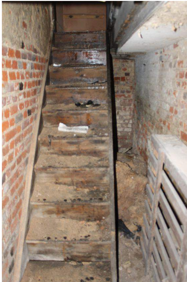
Photograph 41 Staircase leading up from basement of four-storey house (Structure 5). Photograph taken facing north.
