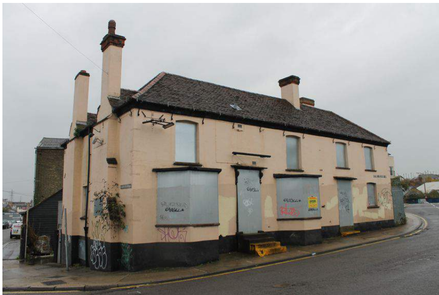
Photograph 5 North-west and north-east elevations of the Rising Sun (left of frame; Structure 1) and the house extension (right of frame; Structure 2). Photograph taken facing south.
