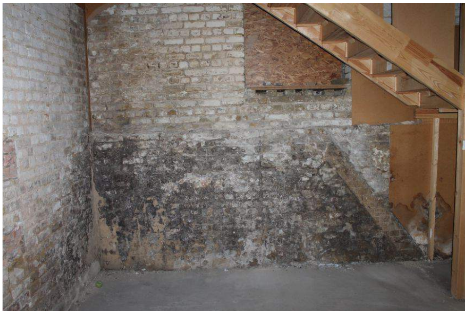
Photograph 86 Visible scarring on brickwork of original staircase in ground-floor of Structure 8. Modern staircase visible to right of frame. Photograph taken facing west.
