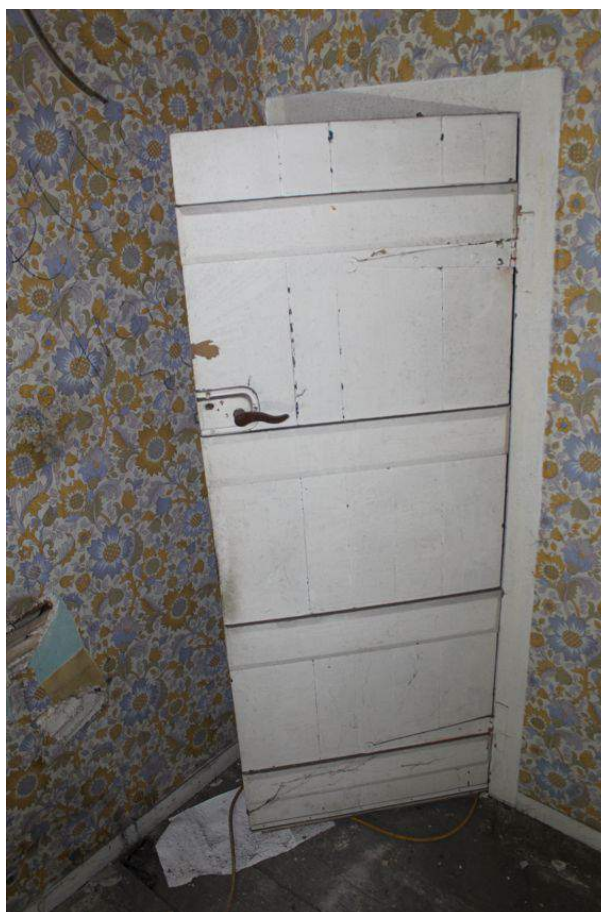
Photograph 33 Rear of vertical-planked door, showing Bakelite handle and rim latch. Photograph taken facing west.
