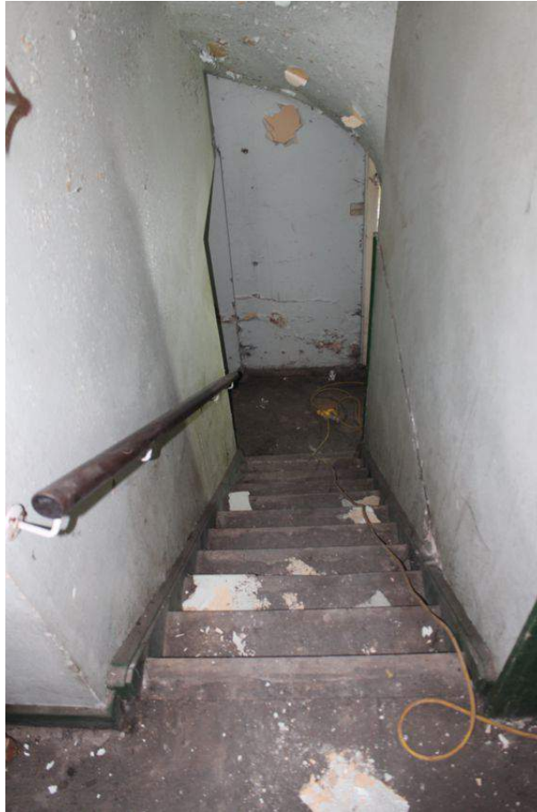
Photograph 12 Staircase leading down to basement from ground-floor of Rising Sun. Photograph taken facing south-east.
