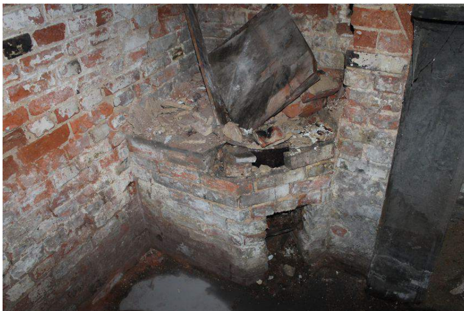
Photograph 44 Brick-built water heater in eastern room of Structure 5's basement adjacent to fireplace. Photograph taken facing north-west.
