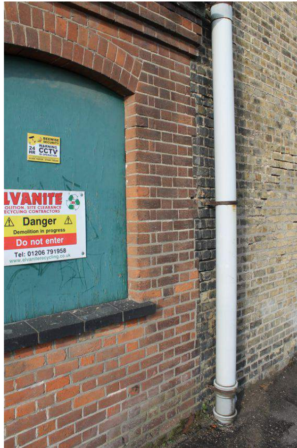
Photograph 94 Detailed shot showing joint between Structures 8 and 9. Alternating brick courses visible due to projecting bricks from Structure 8. Photograph taken facing north-west.
