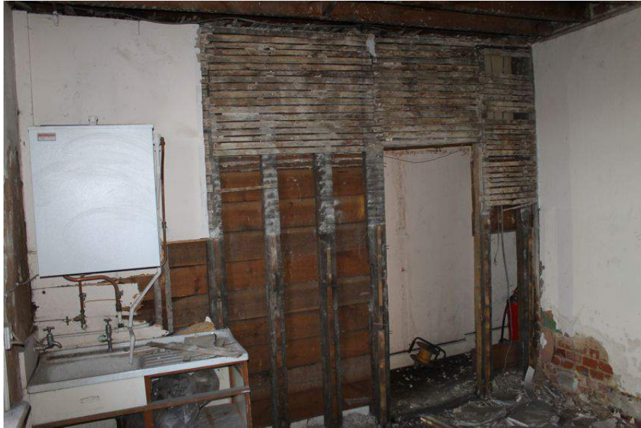
Photograph 46 Exposed lath and plaster wall forming division in ground-floor of Structure 5. Photograph taken facing south-west.
