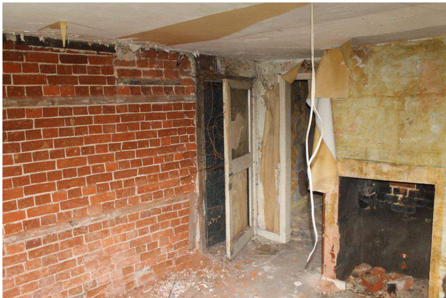
Photograph 28 South-west room on ground-floor of house extension. Showing external entrance, fireplace and exposed brickwork. Photograph taken facing north-west.
