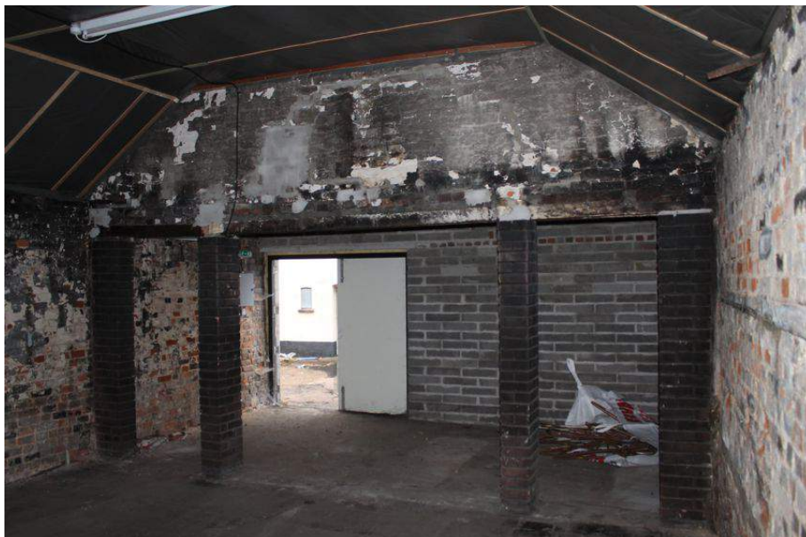
Photograph 35 Internal division within Structure 3, showing brick pillars. Cement block wall visible behind. Photograph taken facing north-west.
