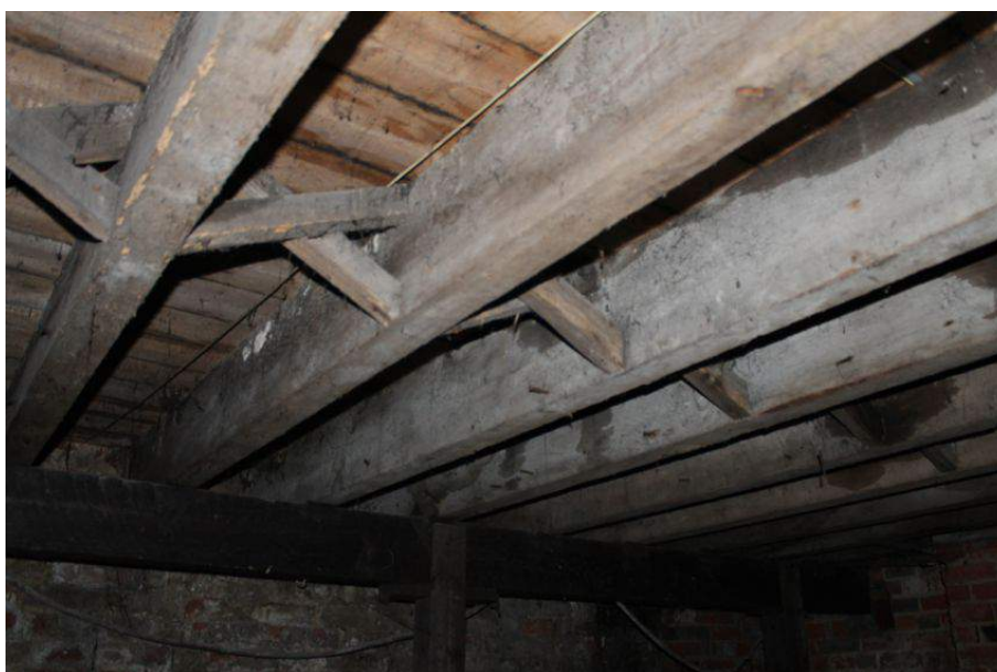
Photograph 45 Herringbone-strutting supporting the ground-floor in the four-storey house. Photograph taken facing north-west.
