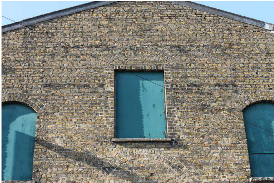
Photograph 55 Upper window in east elevation of Structure 6. Rebuilt brick surround visible. Photograph taken facing west.
