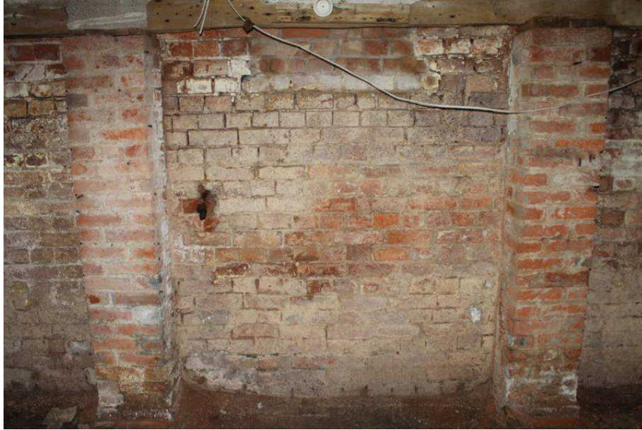
Photograph 23 Detail of wall in northern room of Structure 2's basement, showing inserted brick pillars. Photograph taken facing north-west.
