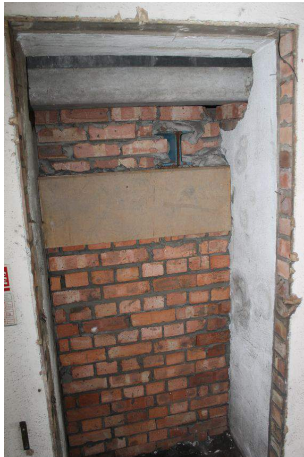
Photograph 49 Blocked entrance from second-floor of Structure 5 into northern warehouse. Metal girder supporting roof of northern warehouse visible. Photograph taken facing south-west.
