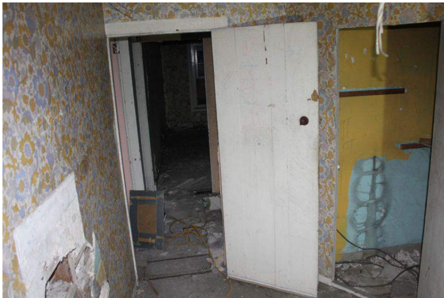
Photograph 32 Vertical-planked door on first-floor of the house extension. Photograph taken facing north-west.
