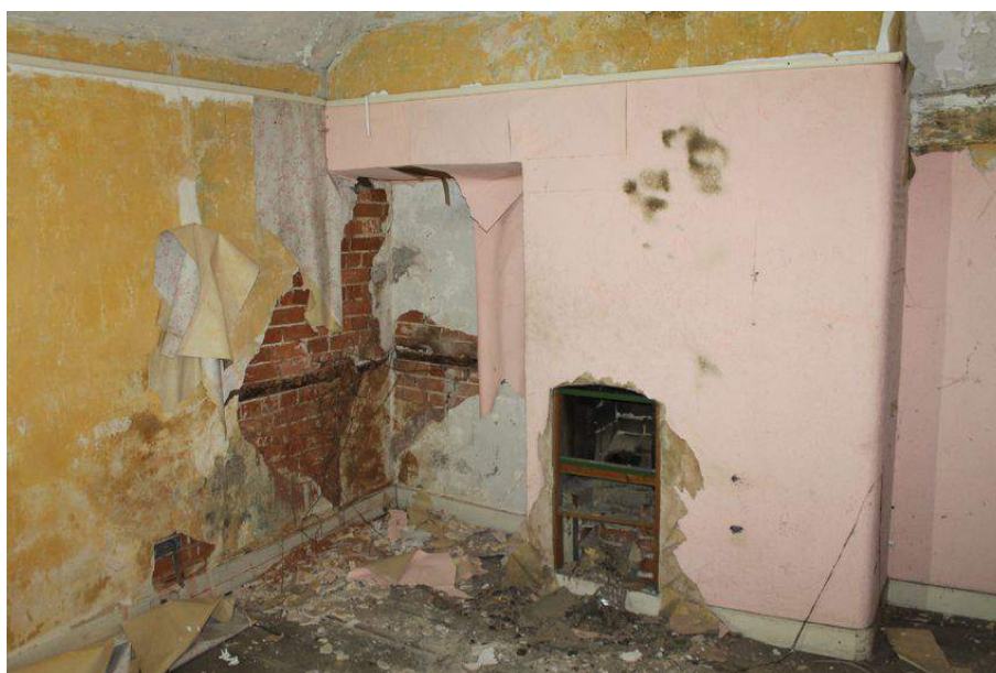
Photograph 31 South-west room on first-floor of Structure 2, showing exposed brickwork and fireplace. Photograph taken facing north-west.
