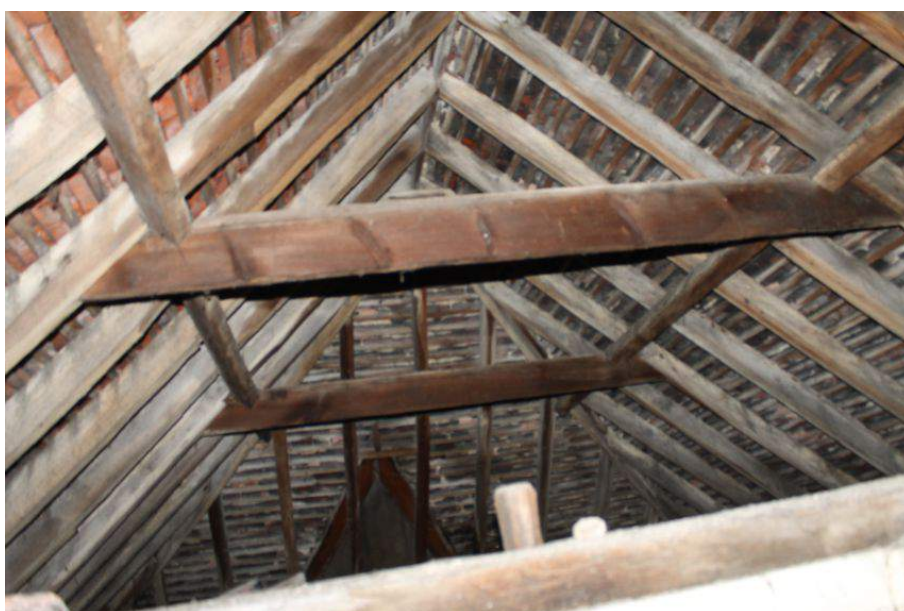
Photograph 19 Roof structure above southern range of Rising Sun, observed from first-floor. Photograph taken facing east.
