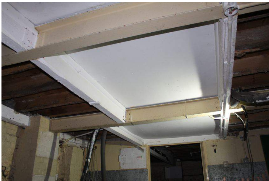
Photograph 11 Modern beams, both timber and metal, supporting the ground-floor of the Rising Sun. Photograph taken facing east.
