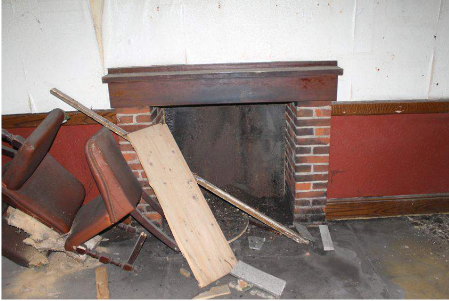
Photograph 16 North-east fireplace on ground-floor of Rising Sun, with modern surround. Photograph taken facing north-east.
