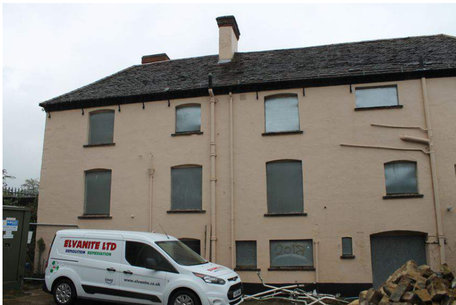
Photograph 7 South-west elevation of the Rising Sun (right of frame; Structure 1) and the house extension (left of frame; Structure 2). Photograph taken facing north-west.
