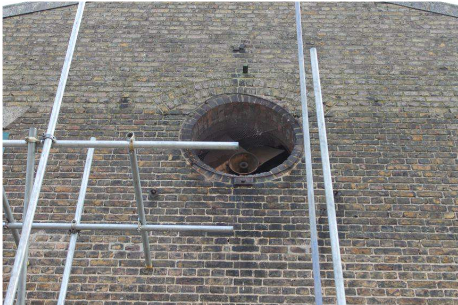
Photograph 70 Inserted metal fan with brick-surround on west elevation of Structure 7. Photograph taken facing east.
