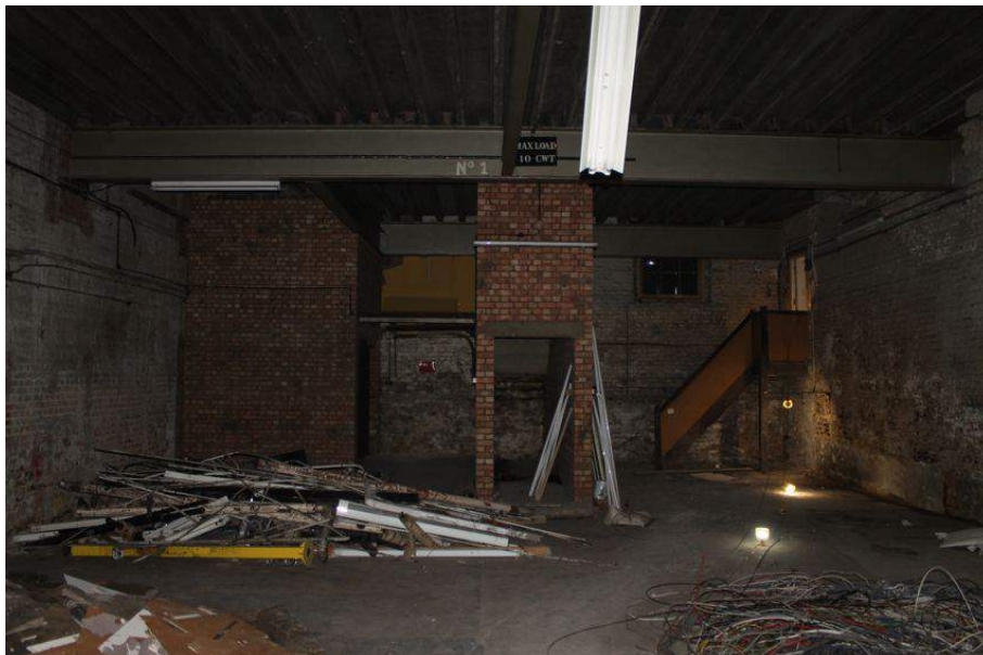
Photograph 59 Inserted modern features in western end of Structure 6's ground-floor. Stairway leading down from first-floor to external door visible in centre. Staircase up to first-floor of Structure 5 visible to right. Photograph taken facing west.
