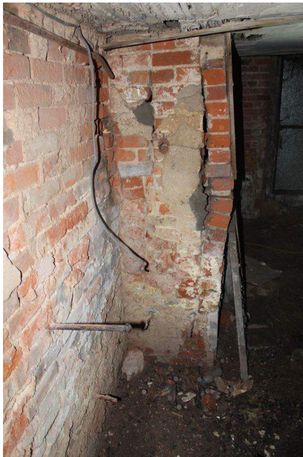
Photograph 24 Eastern side of fireplace in northern room of house extension, showing damage. Photograph taken facing south-west.
