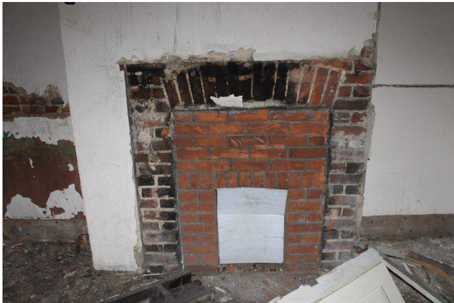
Photograph 47 Partially blocked fireplace in eastern room on ground-floor of Structure 5. Photograph taken facing north.
