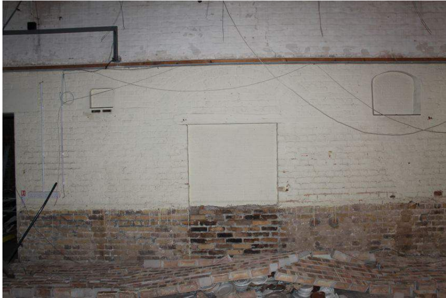
Photograph 62 Original entrance with arch between Structures 6 and 7 at ground-floor level, now bricked over. Photograph taken facing north.
