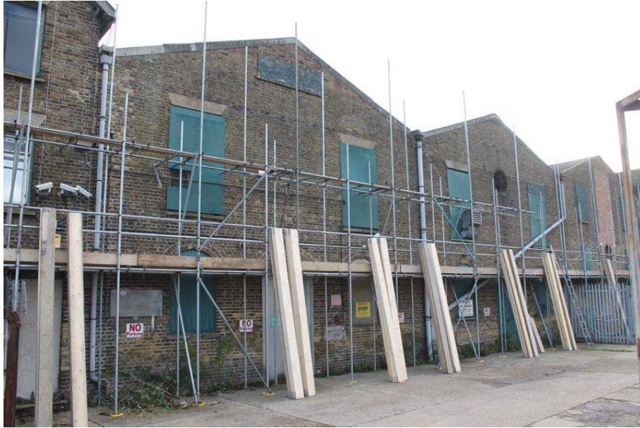
Photograph 56 Western elevation of range of warehouses. Structure 6 to left, Structure 8 to right. Photograph taken facing south-east.
