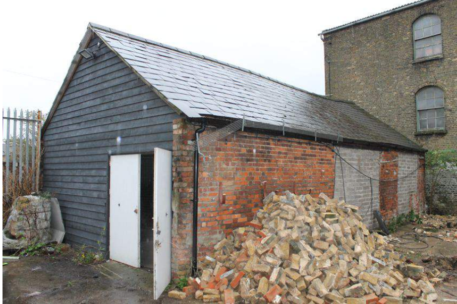
Photograph 34 North-west and south-west elevations of the outbuilding (Structure 3). Photograph taken facing south-east.
