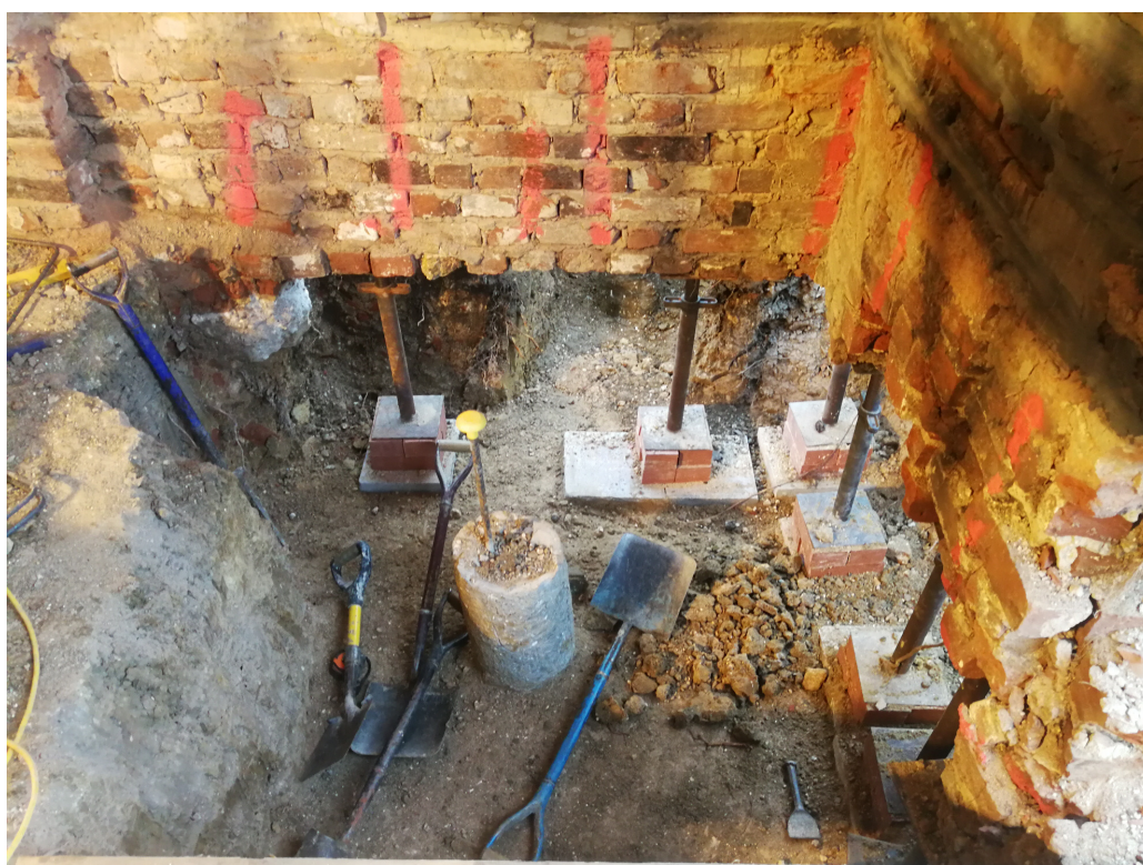
Photograph 6 Excavation of groundbeam slots beneath the extension with temporary props holding up the walls, looking southwest
