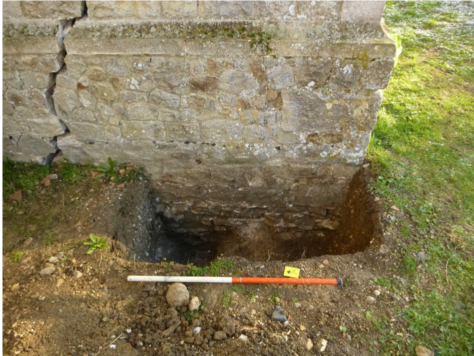
Photograph 1 Test-pit showing foundation of nave and south-west buttress. Substantial crack in wall visible to left. Photograph taken facing east.
