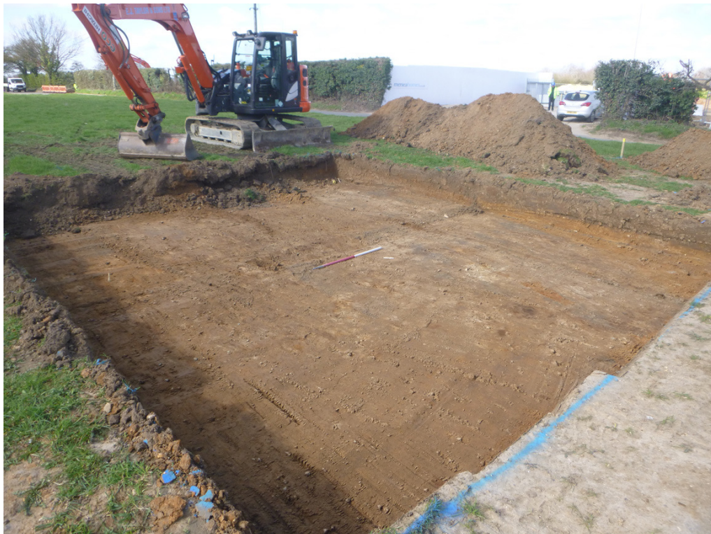
Photograph 1 Site shot of the excavation area for the Flogas tanks, looking west
