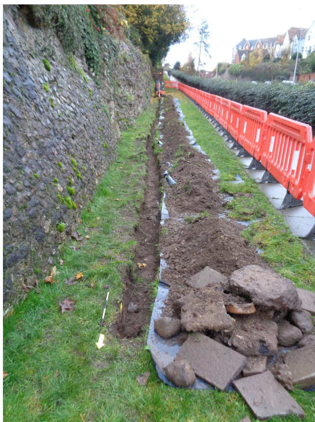
Photograph 5 Phase 2 North of Balkerne Gate - lighting cable trench along Balkerne Hill excavated through L1, looking south.
