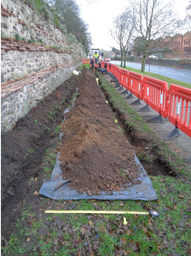
Photograph 10 Phase 2 South of Balkerne Gate - power and lighting cable trenches along Balkerne Hill, looking south.
