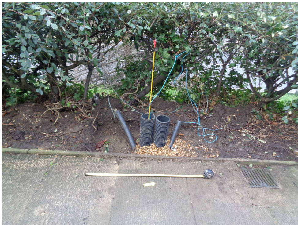
Photograph 7 Phase 2 North of Balkerne Gate – cabinet strip showing central area already backfilled, looking west.
