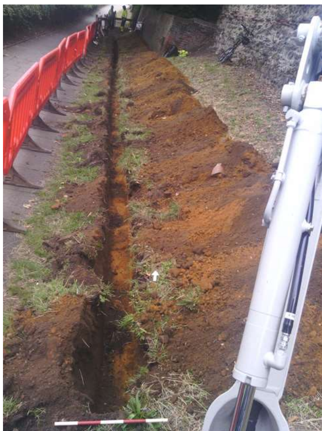
Photograph 4 Phase 1 power cable trench along Balkerne Hill to the north of Balkerne Gate, looking north.
