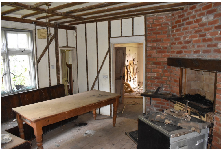
Photograph 14 Interior of room 6, showing timber-framing and rebuilt fireplace. Photograph taken facing north-west.
