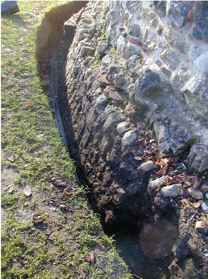
Photograph 7 Collapse of trench wall in T4 (around the chapel) revealing part of the castle wall below ground, looking south
