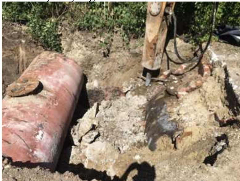
Photograph 1 Petrol tanks and pump
