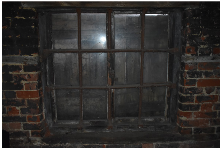
Photograph 13 Original 12-light casement window on north-west elevation, viewed from interior. Iron straps on frame shown. Photograph taken facing north-west.
