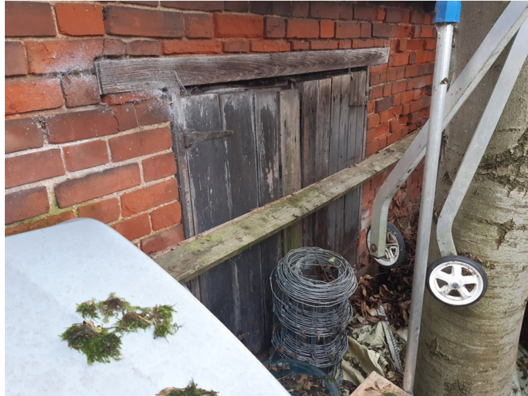
Photograph 4 Detail of shutters of original window on north-west elevation. Photograph taken facing south.
