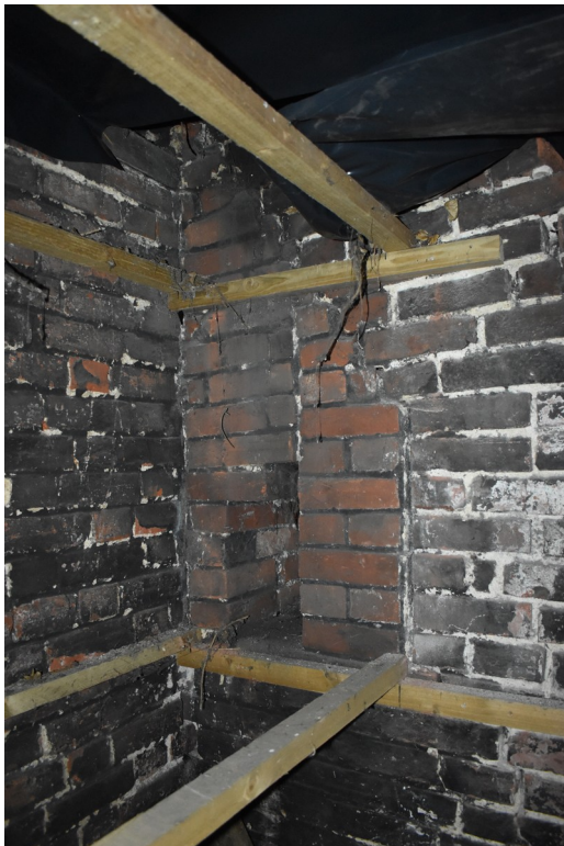
Photograph 7 North-west side of forge, showing more recent bricks bonded in cement mortar. Photograph taken facing east.
