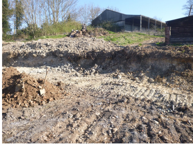
Photograph 2 Recent groundworks to north-east of trench showing extent of terracing. Photograph taken facing north-east.
