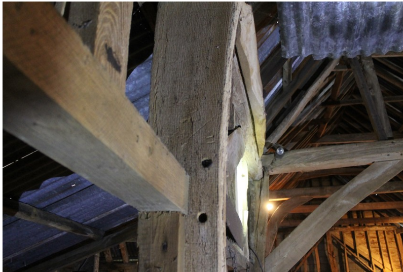
Photograph 11 Detail of carpenter's mark "IV" on northern principal-post between bays 2 and 3. Photograph taken facing east.
