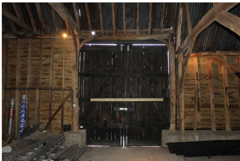
Photograph 14 Detail of barn doors in southern elevation of bay 4. Photograph taken facing south-west.
