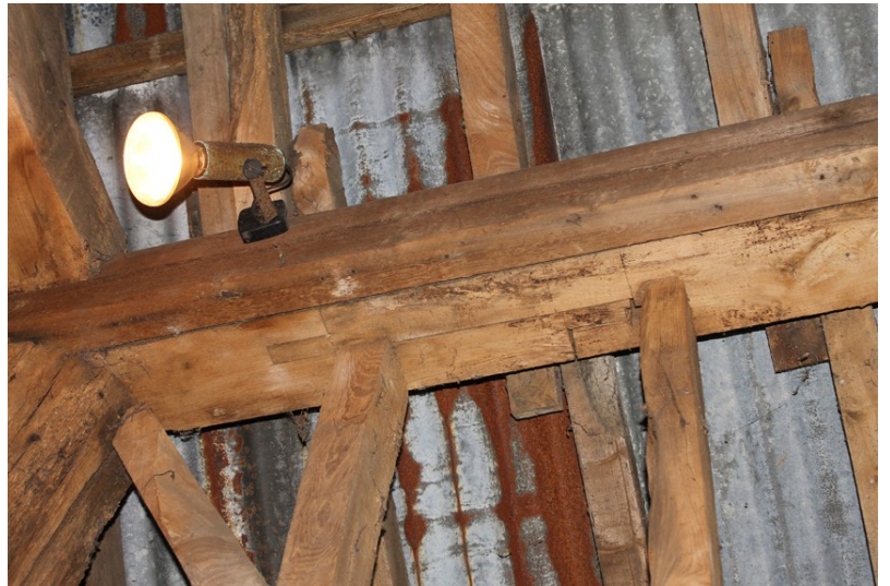
Photograph 17 Detail of scarf joint on northern wall-plate of bay 5. Photograph taken facing north.
