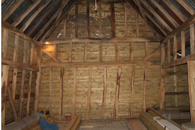
Photograph 6 Western elevation of barn (in bay 1). Re-used sill beam with empty mortices visible. Wind-braces visible in roof above. Photograph taken facing north-west.
