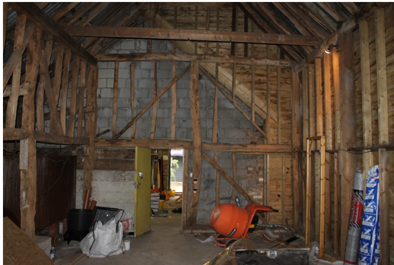
Photograph 18 Eastern end of barn (in bay 6), with re-used timber. Photograph taken facing south-east.
