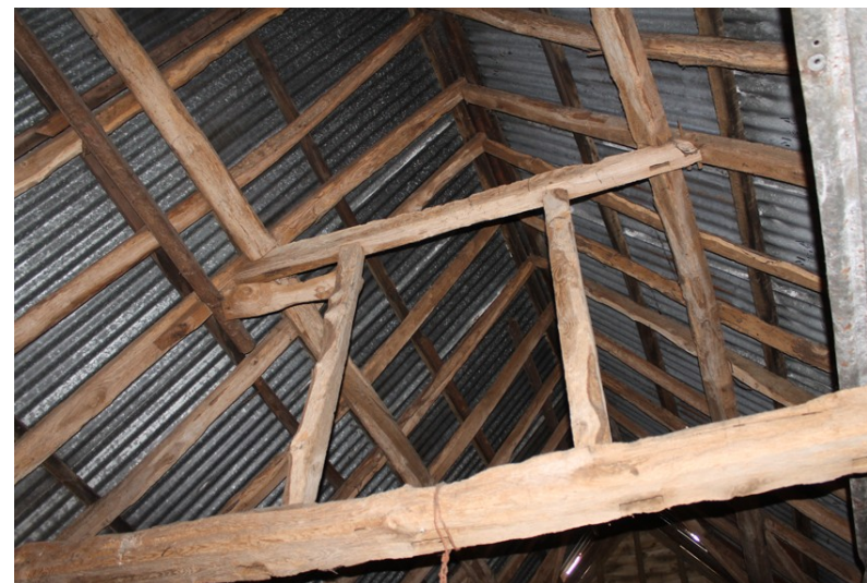
Photograph 8 Detail of underside of collar between bays 1 and 2, showing empty mortices at each end, adjacent to queen-struts. Photograph taken facing east.
