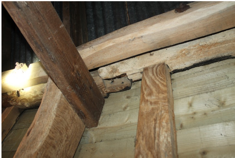
Photograph 12 Detail of partially sprung scarf joint in southern wall-plate of bay 2. Photograph taken facing south.
