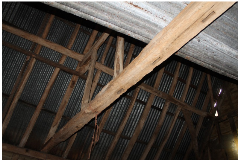
Photograph 7 Detail of underside of tie-beam between bays 1 and 2, showing empty mortices. Photograph taken facing south-west.
