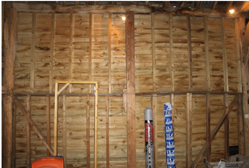
Photograph 15 Southern elevation of bays 5 and 6, showing rebuilding using modern machine-cut timber. Photograph taken facing south-west.
