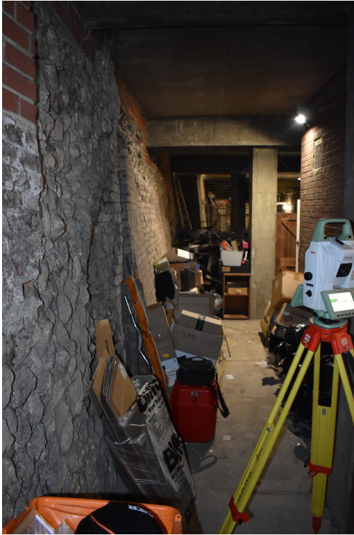
Photograph 5 Oblique shot of section 6 behind St John's Street, showing re-used septaria and wall to the east. Photograph taken facing north-east.
