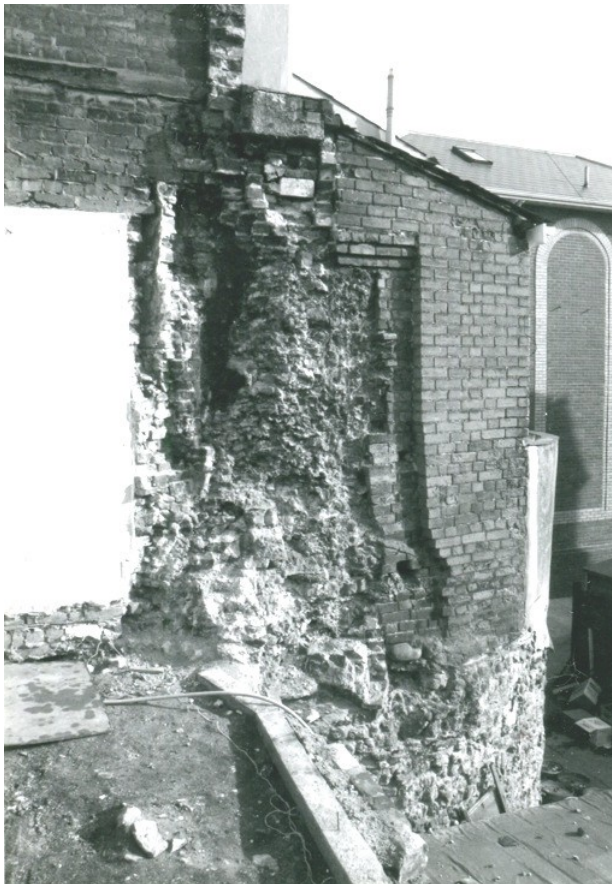
Photograph 1 1988 photograph showing the western side of bastion 6, with modern brick-built structure on top. Photograph taken facing south-east.
