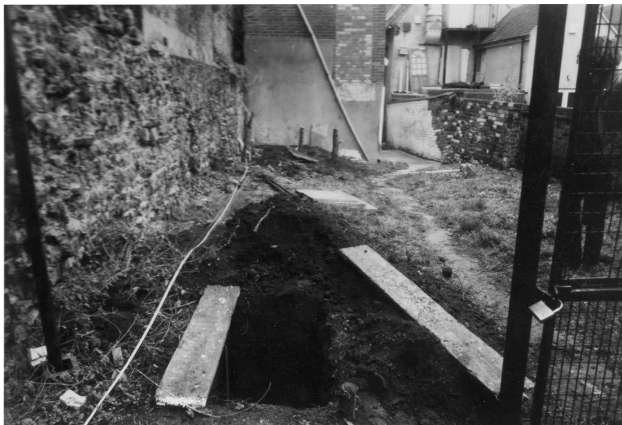
Photograph 3 Site shot showing excavation of test-pits adjacent to section 8 of town wall in 1991. Photograph taken facing east.
