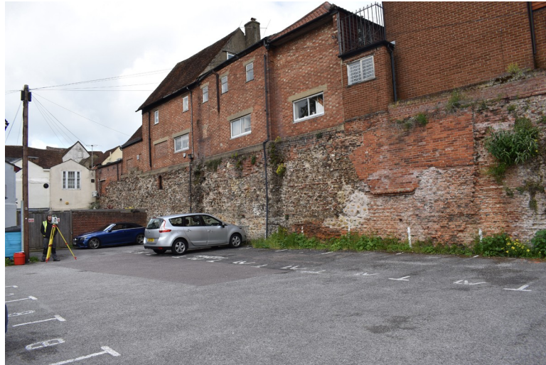
Photograph 9 Western end of section 7, showing medieval refacing along with modern brickwork. Photograph taken facing north-west.
