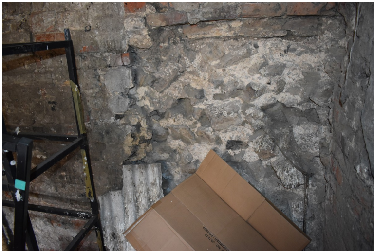
Photograph 8 Detail of exposed area of septaria and mortar core in section 6. Photograph taken facing north.
