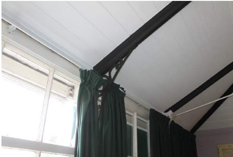
Photograph 31 Detail of metal braces supporting roof of conservatory. Photograph taken facing west.
