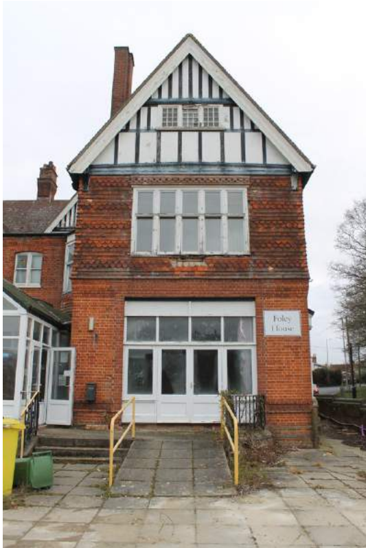
Photograph 8 Detail of eastern-wing on south-west elevation. Replacement windows and brickwork visible on ground-floor. Photo taken facing north-east.
