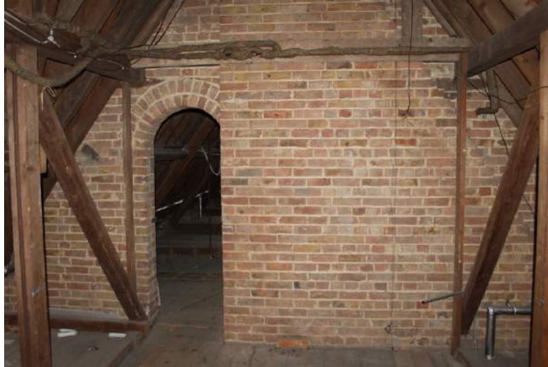
Photograph 36 Room 91, showing entrance into room 90 and chimney-stack rising from floors below. Photograph taken facing south-west.
