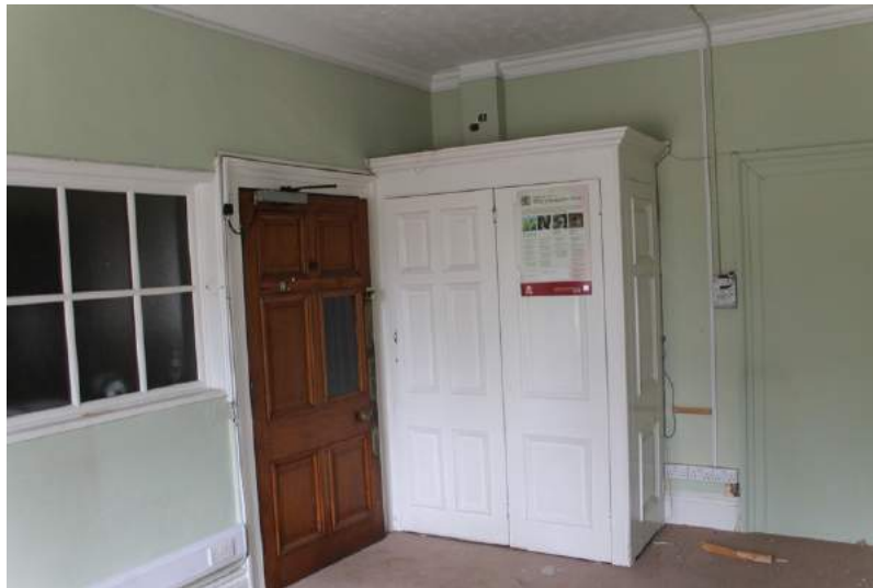
Photograph 26 Detail of original cupboard in room 15, along with inserted window to left of frame and blocked window to right. Photograph taken facing south.
