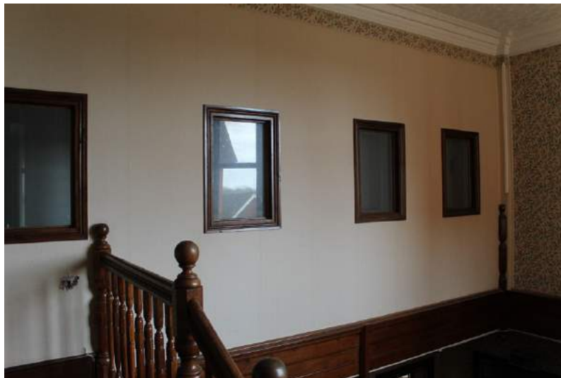
Photograph 35 Modern wall inserted on landing above main staircase, with windows. Note newel post to right of frame from original railing. Photograph taken facing south.
