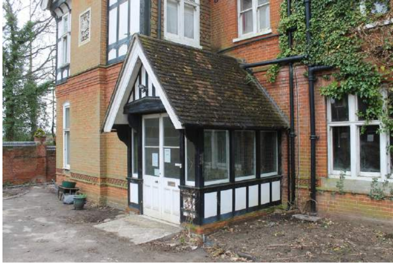
Photograph 12 Detail of porch projecting from north-east elevation, with stained-glass windows visible. Photograph taken facing south.
