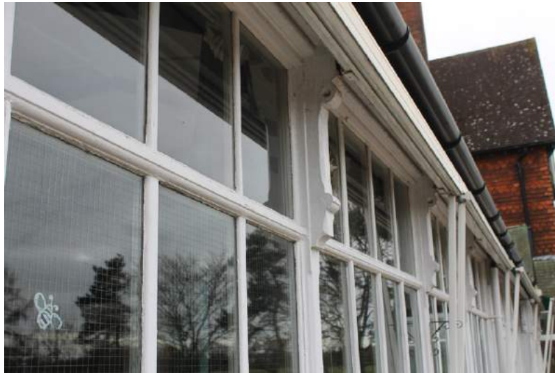
Photograph 5 Detail of corbels at top of mullions between windows on conservatory on south-west elevation. Modern safety glass visible on middle panes, original plate glass visible on upper panes. Photograph taken facing east.
