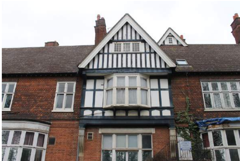
Photograph 10 Detail of central projecting imitation timber-framed bay with oriel window on south-east elevation. Inserted modern door visible to right of bay. Photograph taken facing north-west.
