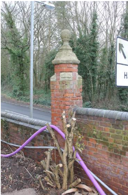
Photograph 3 Brick pillar and stone corbel at original end of boundary wall surrounding Foley House. Modern inserted brick wall to left of frame. Photograph taken facing east.
