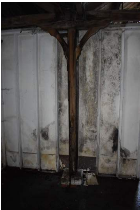
ECC4613_Photograph_067 Original unpainted post in Room 1, against modern inserted stud wall - view north-east.
