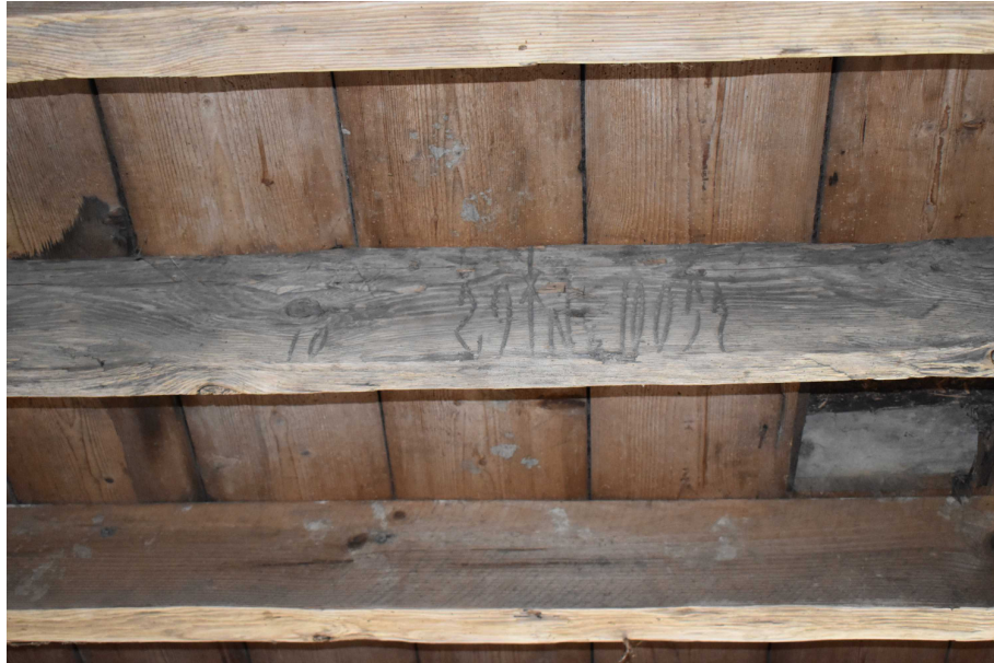
Photograph 15 Detail of Baltic timber mark on joist supporting the first floor of Room 1 - view east.
