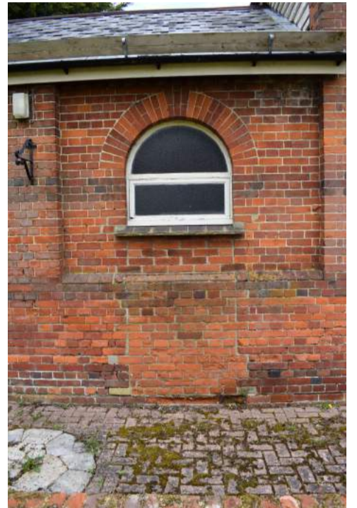
ECC4613_Photograph_006 Detail of blocked doorway with modern window on southern elevation of the main range to the coach house.
