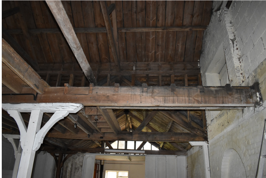
Photograph 19 Cut joists in the flooring of Room 6 - view west.
