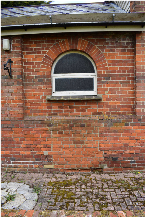
Photograph 3 Detail of blocked doorway with modern window on southern elevation of the main range – view north.
