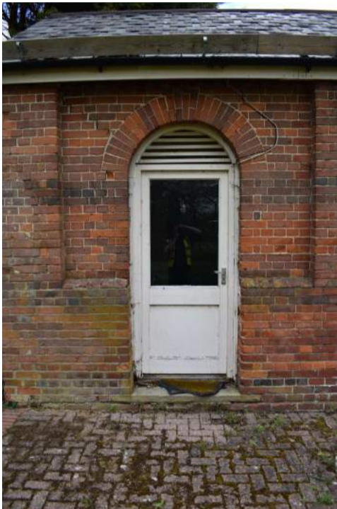
ECC4613_Photograph_005 Detail of modern door on southern elevation of main range to the coach house.
