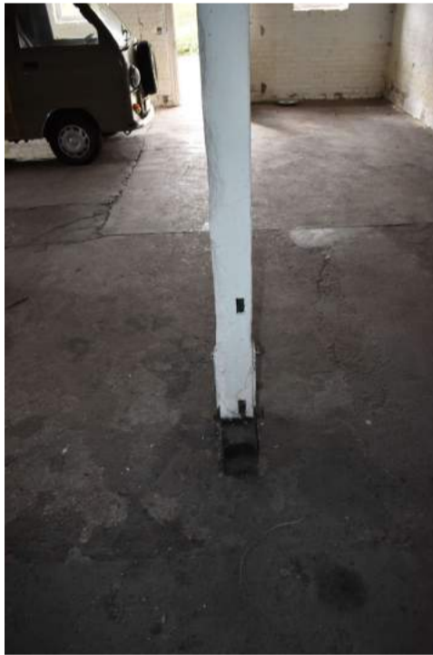
ECC4613_Photograph_092 Detail of mortices in base of post in Room 1 - view south.
