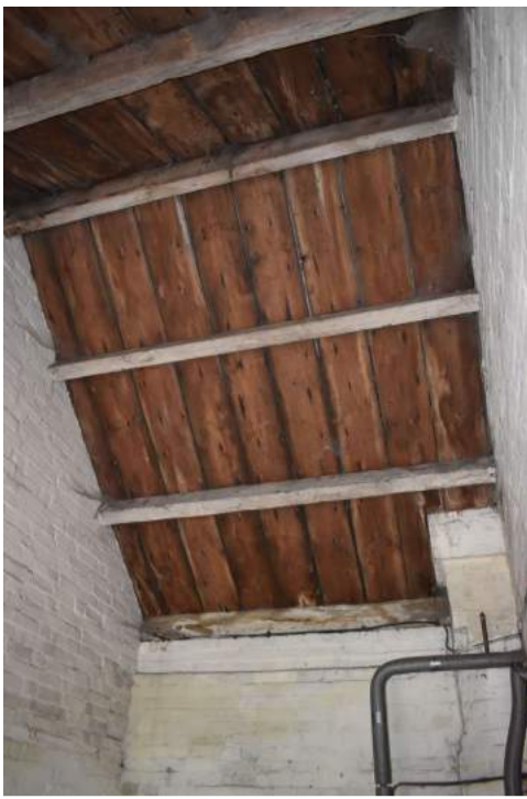
ECC4613_Photograph_085 Northern roof pitch of Room 2, with Baltic timber marks - view north-west.
