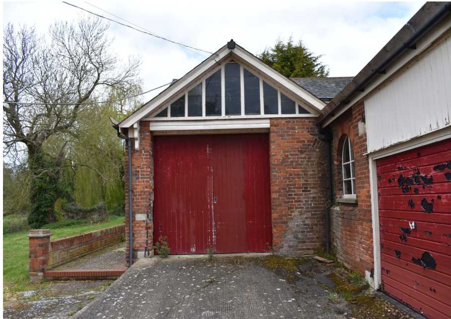
Photograph 8 East elevation of the main range with an original stable door and second original opening compromised by later alterations – view west.
