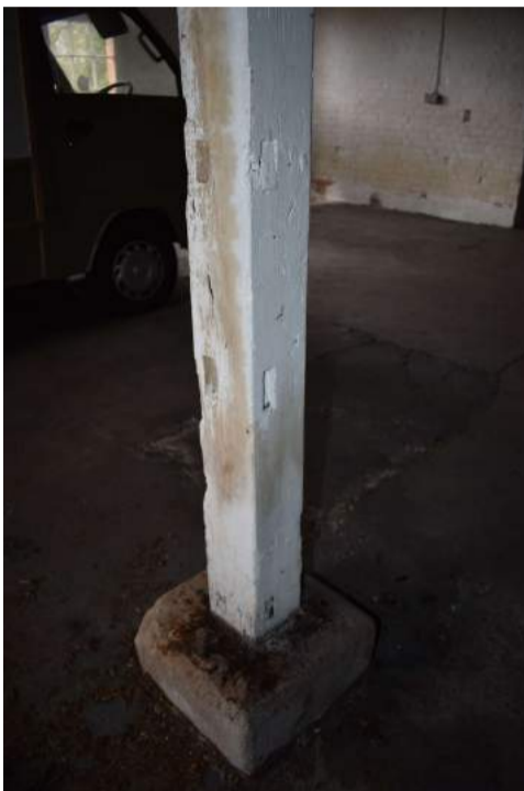
ECC4613_Photograph_065 Empty mortices on post in Room 1, would have originally supported division.
