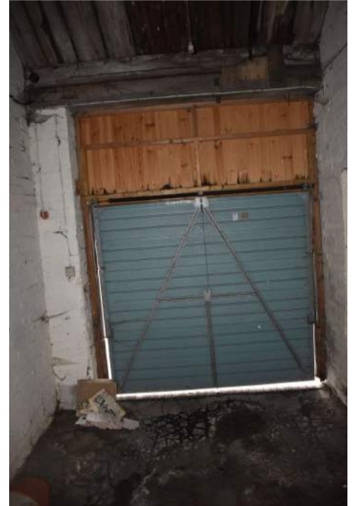
ECC4613_Photograph_090 Modern inserted stud wall and garage door in southern wall of Room 3 - view east.
