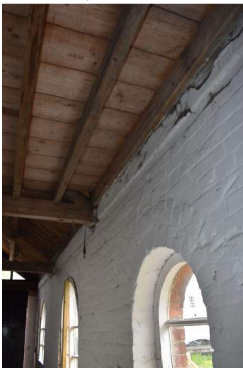
ECC4613_Photo... Location of Baltic timber mark on joist of Room 6 - view south-east.
