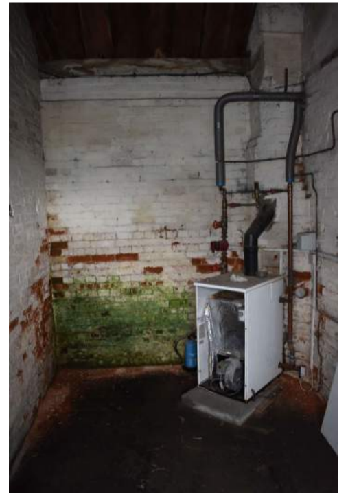
ECC4613_Photograph_081 Room 2, showing original fireplace to right with modern boiler in front - view...
