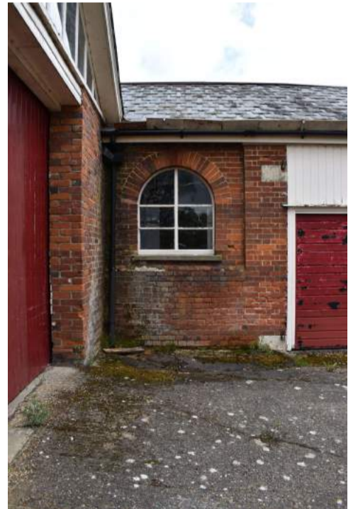
ECC4613_Photograph_009 Original window on southern elevation of the secondary range to the coach house.
