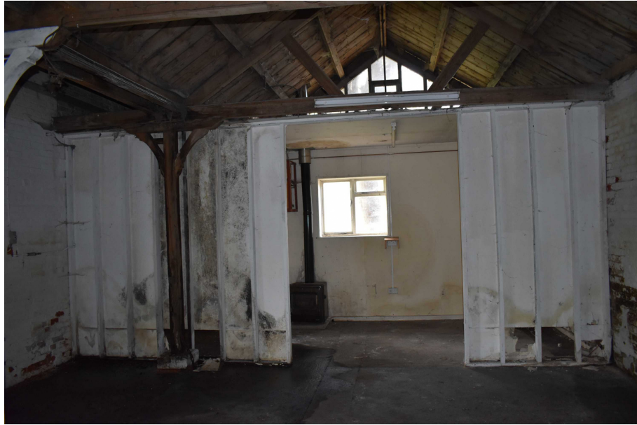
Photograph 17 Detail of inserted stud wall and original post in western end of Room 1 - view west.
