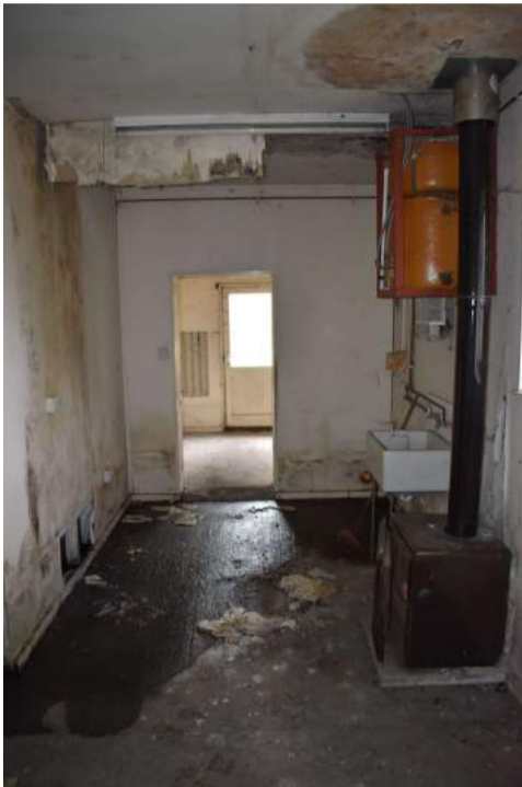
ECC4613_Photograph_077 Room 1a, in area converted to house a boiler (right of frame) - view south.
