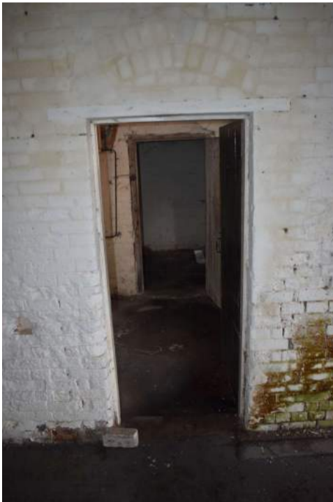
ECC4613_Photograph_080 Original doorway, with later frame, leading into Room 2 from Room 1 - view...
