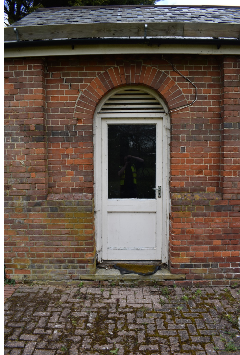
Photograph 4 Detail of modern door in original opening on the south elevation of the main range - view north.
