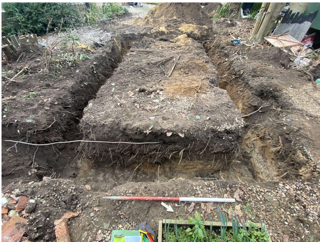
Photograph 2 General view of footings from NE end, looking SW. Copper oil pipes can be seen running right to left in the foreground of the photograph.
