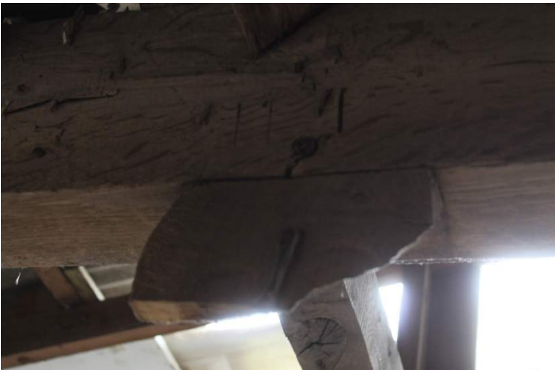
Photograph 12 Carpenter's mark on tie-beam T3 above the remains of an inserted post to support the loft.
