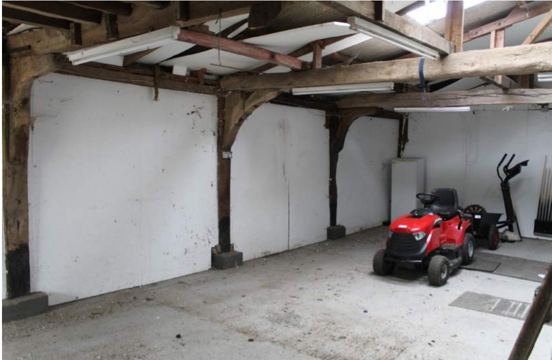
Photograph 4 Interior of the cart lodge showing the south wall with its exposed posts and protective concrete shoes – view south-west.
