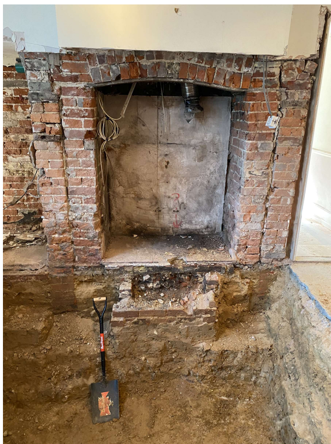
Photograph 3 The grand hall fireplace showing additional brickwork inside to narrow the opening and part of the brick structure to the front, looking south
