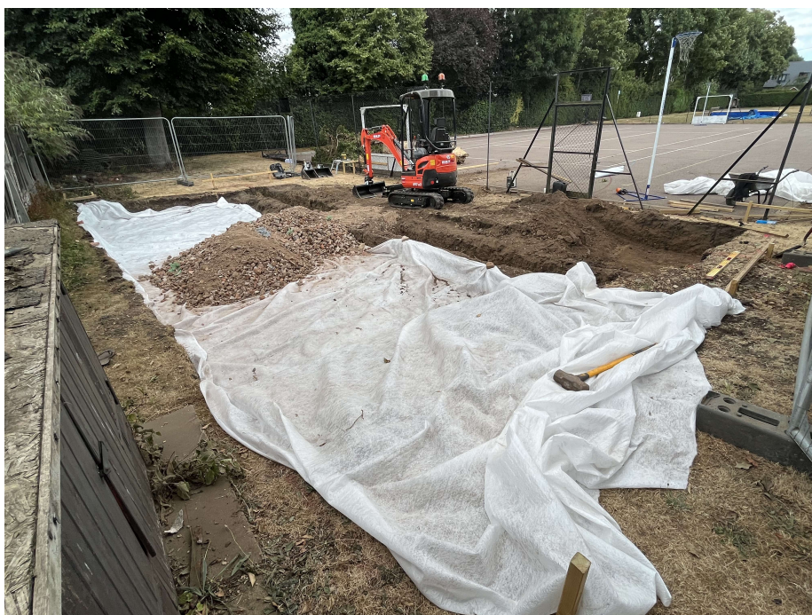
Photograph 4 General view of site from south-west corner of site with Pad 3 strip in background, looking north-east
