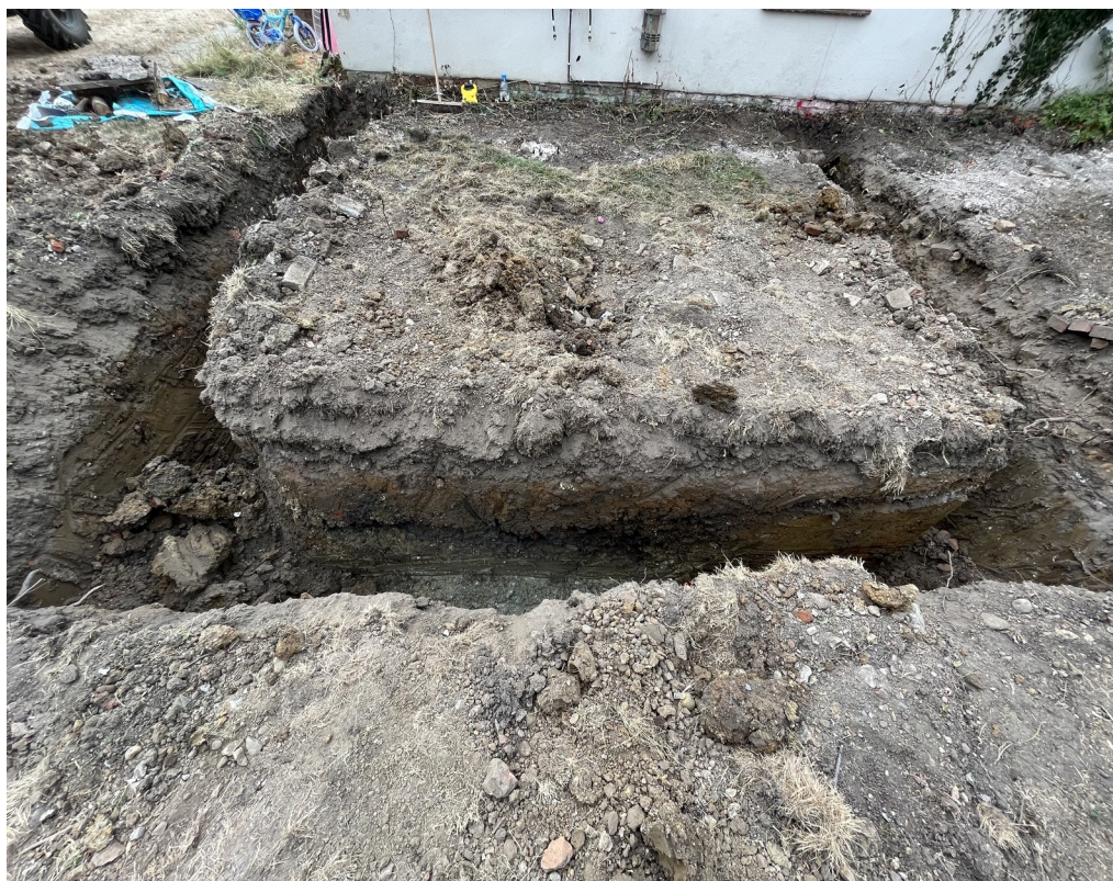
Photograph 2 The main foundation trench from the north side, showing F1 in section, looking south.
