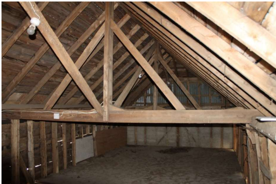
Photograph 15 Detail of one of the tie-beams which have both lateral and longitudinal bracing to the king post - view south-east
