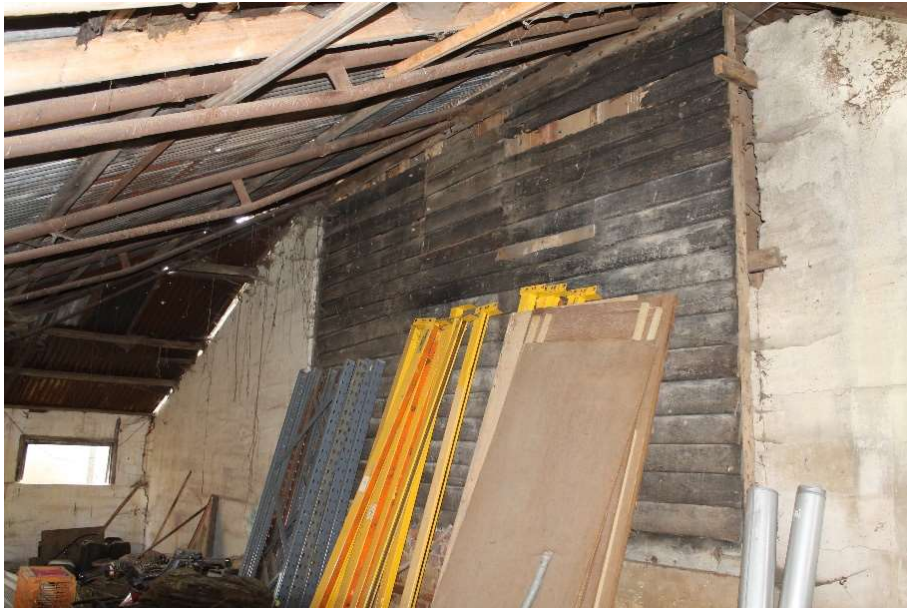
Photograph 10 Extension C with the weatherboard of the barn in the centre of the picture – view south-east
