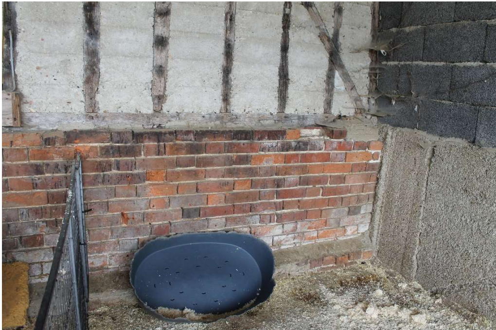
Photograph 6 Detail of the dwarf wall and plinth of the barn with infilled timber frame visible above – view west
