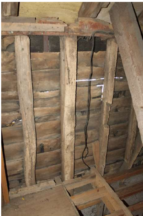
Photograph 16 Detail of the north-east frame showing machine-cut timbers next to hand-sawn and re-used timbers.
