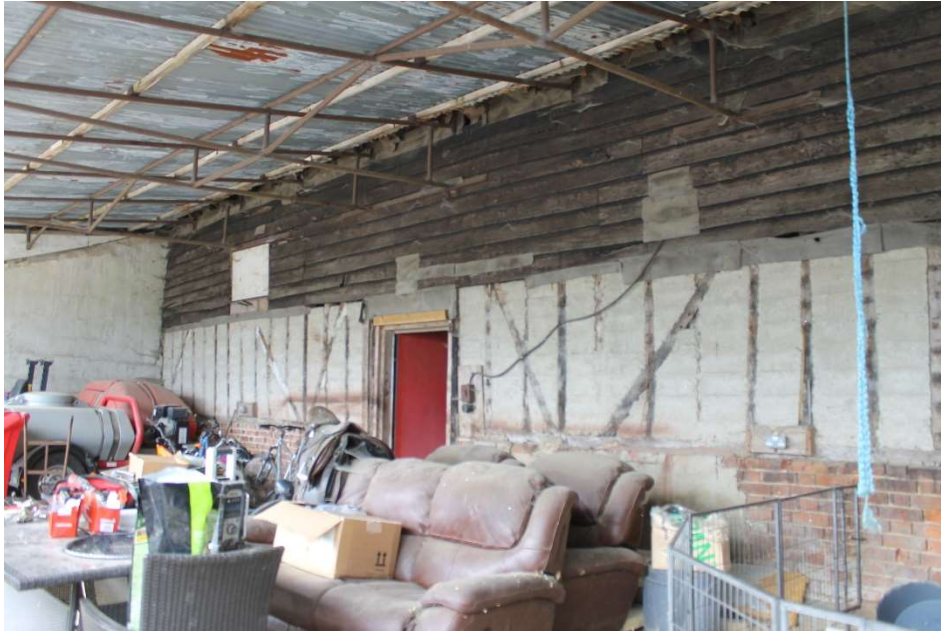
Photograph 5 Extension D, the covered external yard showing the brick plinth and timber frame of the barn – view south
