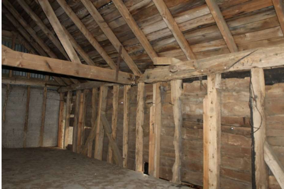
Photograph 14 Common rafters rising from the wall-plate with sarking boards above and one of the tie-beams, which do not correspond with a principal post - view south
