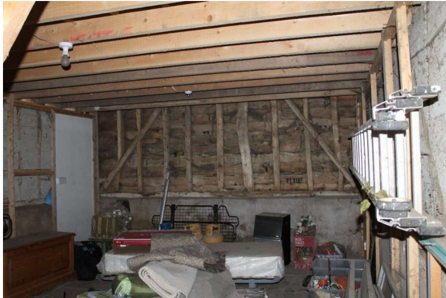
Photograph 12 Interior of the barn showing the surviving timber frame of the north-west wall – view north-west
