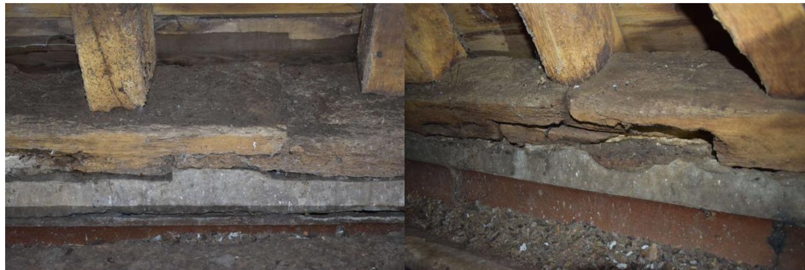
SOWBF22_PhotoGraph_063Detail of cement-filled mortices on sill-bea... SOWBF22_PhotoGraph_064Detail of timber frame in store 4. Photogra...
