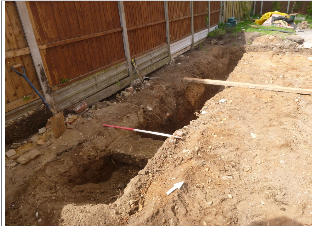
Photograph 3 Trenching in west corner of site with concrete footing, looking north west.
