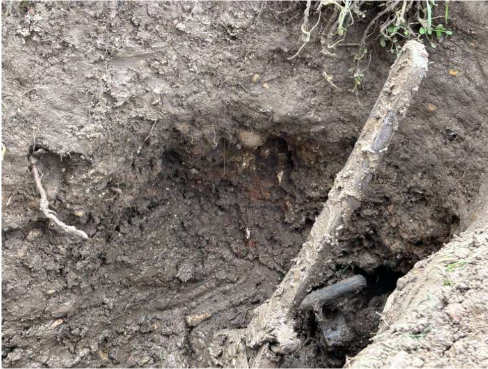
Photograph 3 Close-up of suspected backfill underneath church footings, view south-east.
