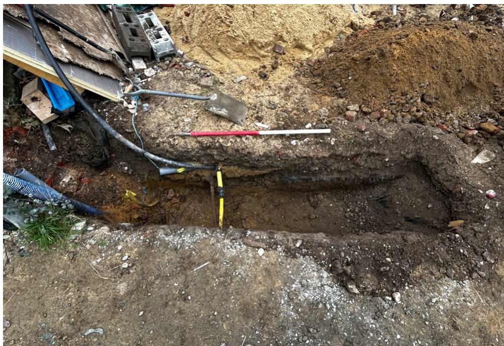
Photograph 13 The northern end of the foundations for the new wall. View east.
