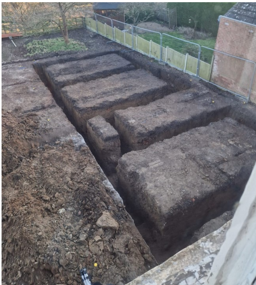
Photograph 3 New dwelling foundations excavated for the first time, prior to concreting. View south. Photo taken by Crosbys Building Contractors Ltd.
