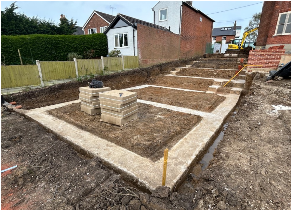
Photograph 1 Working shot of the south-east end of new dwelling foundations. View west.
