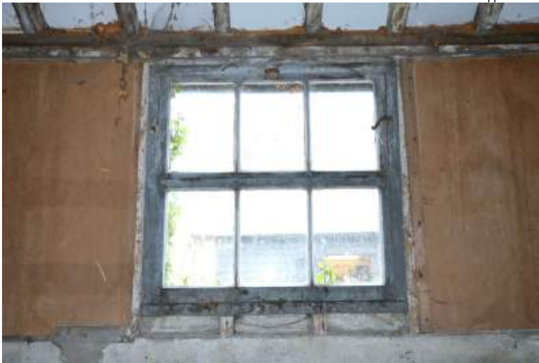
MGWF24_PhotoGraph_017 Interior shot of timber framed window of cowshed, bay 4. Photograph taken facing east.
