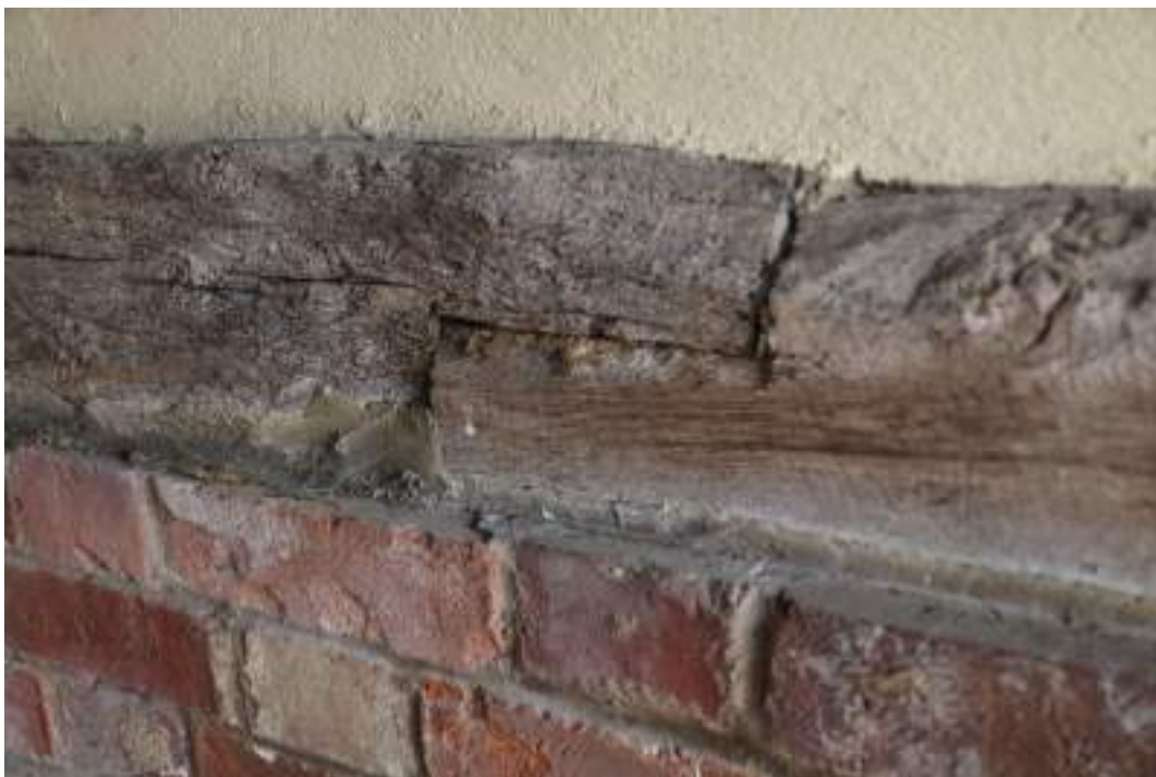
MGWF24_PhotoGraph_091 Interior detail shot of side-halved scarf-joint of sill-beam in carport. Photograph taken facing south-east.
