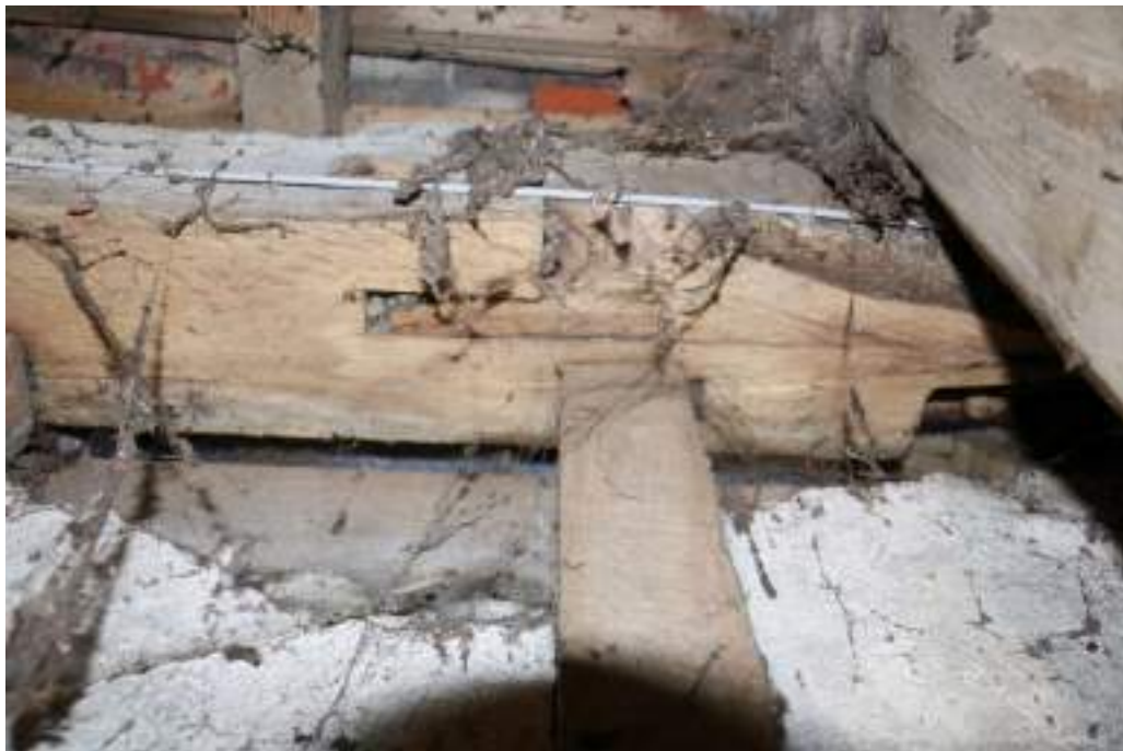
Photograph 9 Detail of scarf-joint in wall-plate of bay 1 of threshing barn. Photograph taken facing west.
