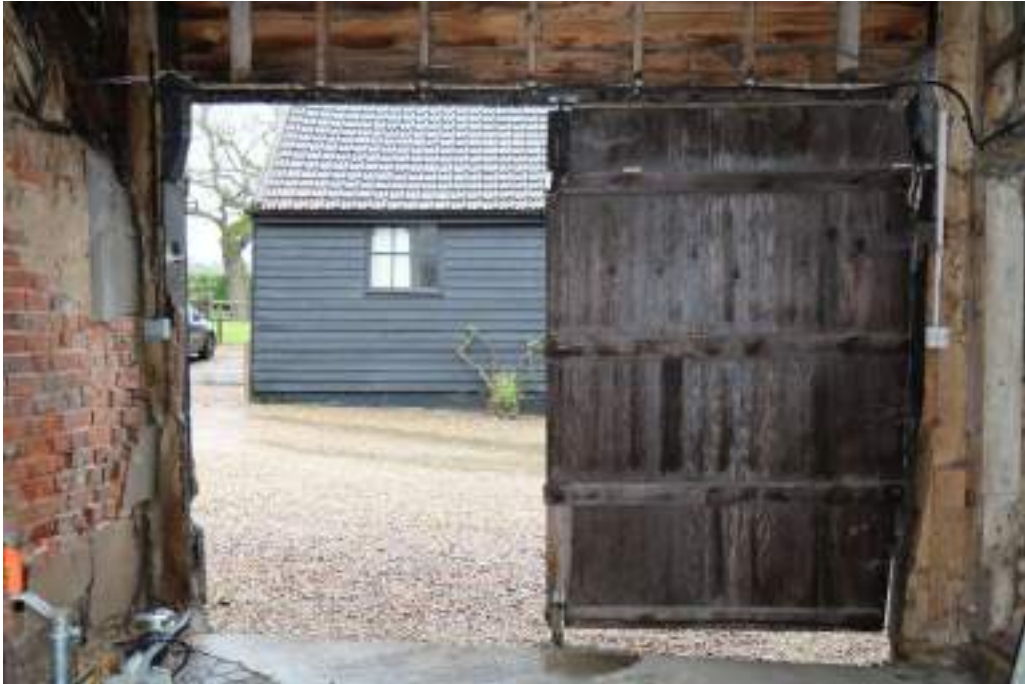
Photograph 15 Detail of doorway in midstrey of threshing barn. Photograph taken facing west.
