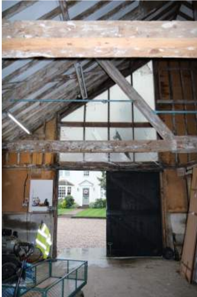
Photograph 33 Detail of doors and windows in bay 1 of cowshed. Photograph taken facing south.
