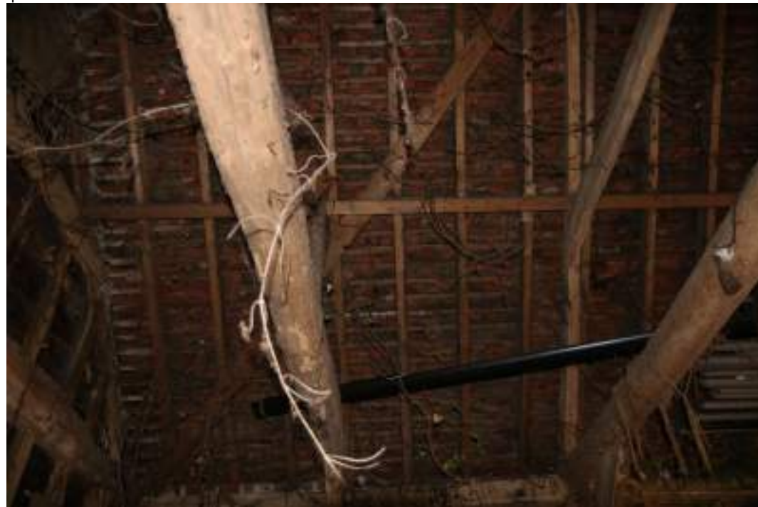
MGWF24_Phograph_118 Interior detail shot of roof construction in bay 1 of threshing barn. Photograph taken facing east.
