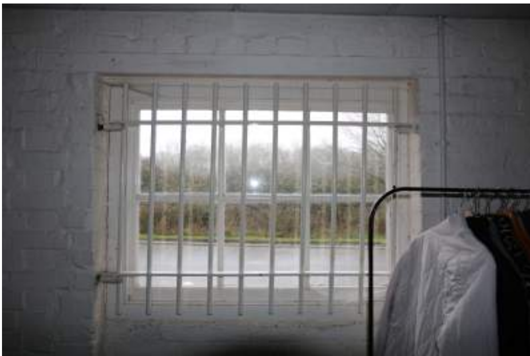
MGWF24_PhotoGraph_031 Interior detail shot of timber framed window in brick building, room 1. Photograph taken facing north.
