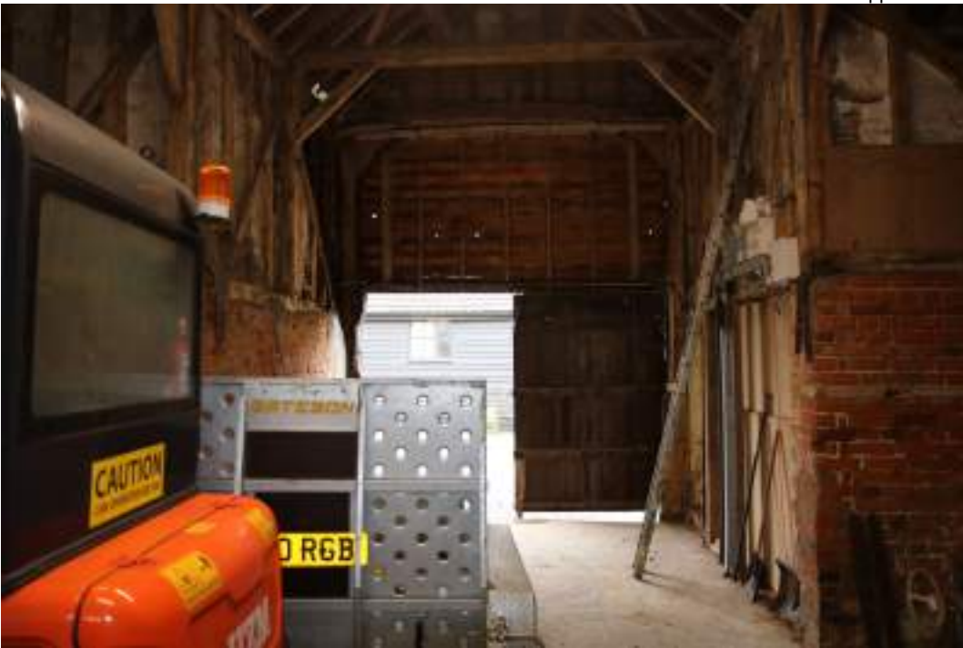
MGWF24_Phograph_133 Interior shot of bay 3 and midstrey of threshing barn. Photograph taken facing west.
