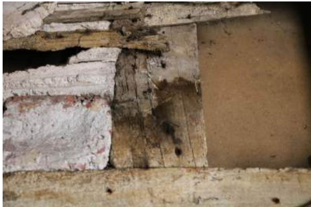
MGWF24_PhotoGraph_080 Interior detail shot of carpenter's mark on stud in lean-to 2. Photograph taken facing east.
