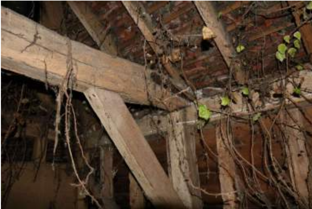
Photograph 10 Detail of inserted tie-beam with straight brace and iron strap, in bay 1 of threshing barn. Photograph taken facing north-east.
