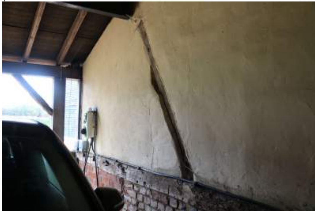
MGWF24_PhotoGraph_098 Interior detail shot of wind-brace in carport. Photograph taken facing north-west.
