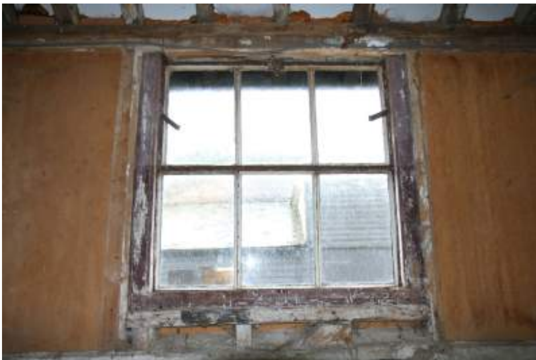
MGWF24_PhotoGraph_011 Interior detail shot of inserted metal framed window in cowshed, bay 3. Photograph taken facing east.
