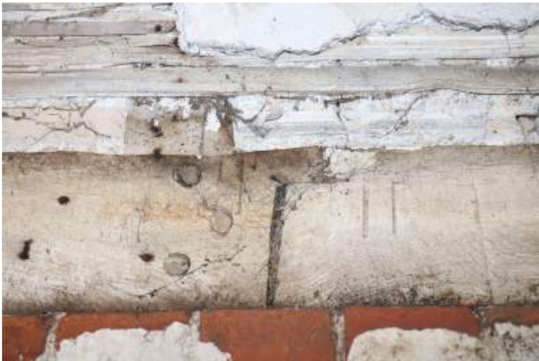
MGWF24_PhotoGraph_079 Interior detail shot of scarf-joint and carpenter's marks on sill-beam of lean-to 2. Photograph taken facing north.
