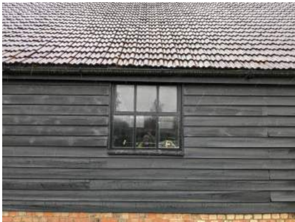
MGWF24_PhotoGraph_191 Detail shot of window in western elevation of cowshed. Photograph taken facing east.
