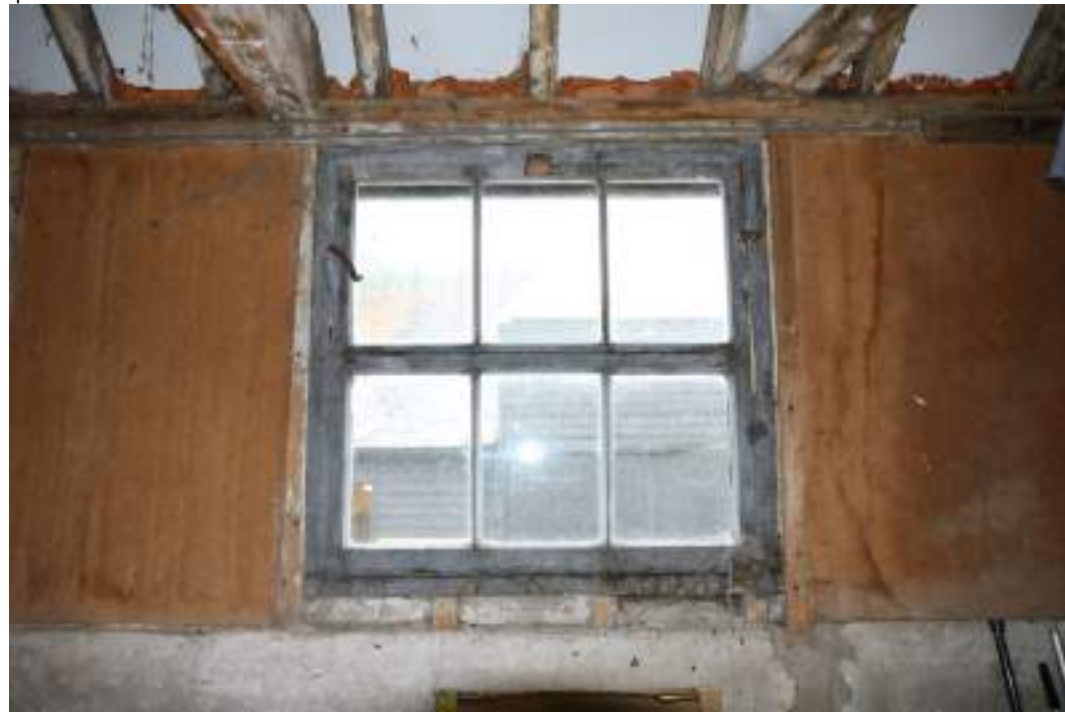
MGWF24_PhotoGraph_010 Interior detail shot of timber framed window in cowshed, bay 2. Photograph taken facing east.
