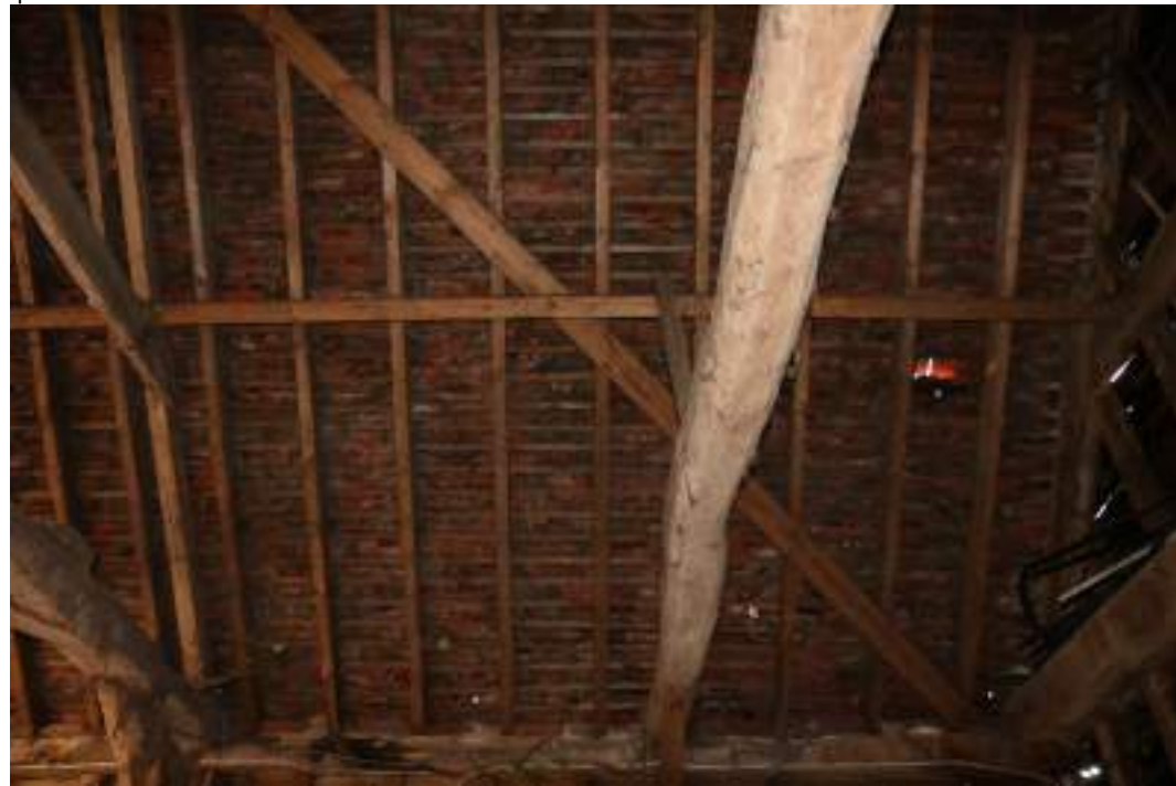
MGWF24_PhotoGraph_146 Interior detail shot of roof construction in bay 4 of threshing barn. Photograph taken facing east.
