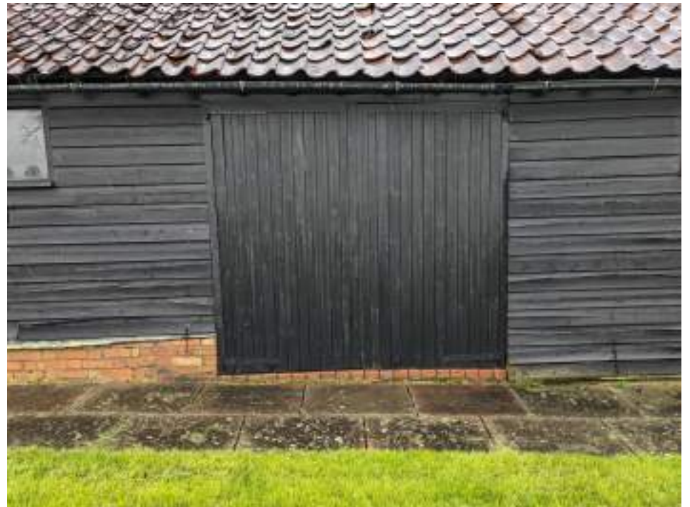
MGWF24_PhotoGraph_196 Detail shot of doors in southern elevation of small barn. Photograph taken facing north.
