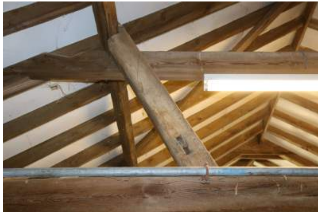
MGWF24_Phograph_064 Interior detail shot of reused timber inclined strut between bays 3 and 4 in small barn. Photograph taken facing west.
