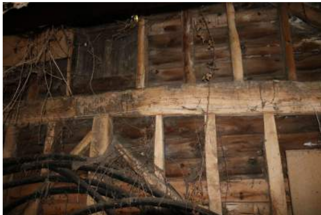
MGWF24_Phograph_120 Interior detail shot of reused timber tie-beam in bay 1 of threshing barn. Photograph taken facing north.
