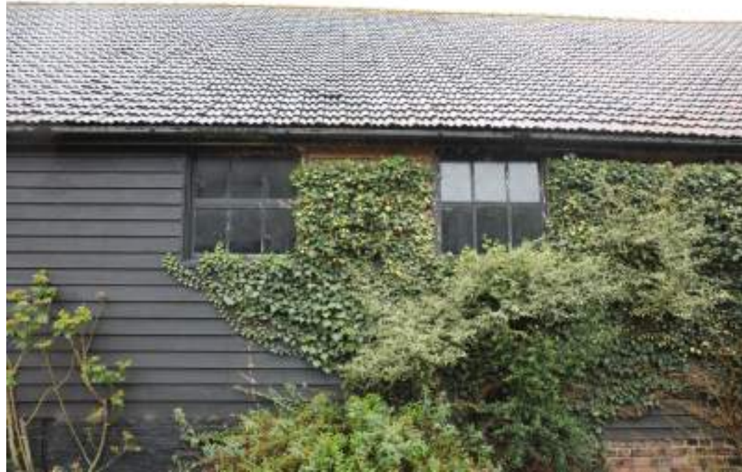
MGWF24_PhotoGraph_186 Detail shot of windows on western elevation of cowshed. Photograph taken facing west.
