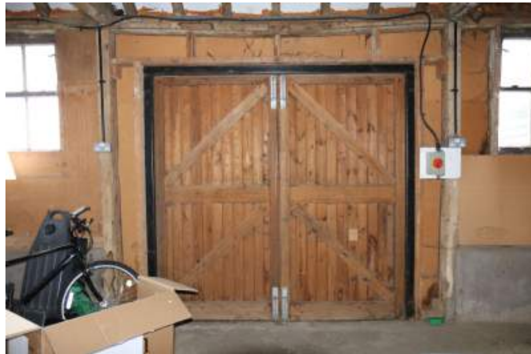
MGWF24_PhotoGraph_020 Interior detail shot of replacement door in cowshed, bay 5. Photograph taken facing west.
