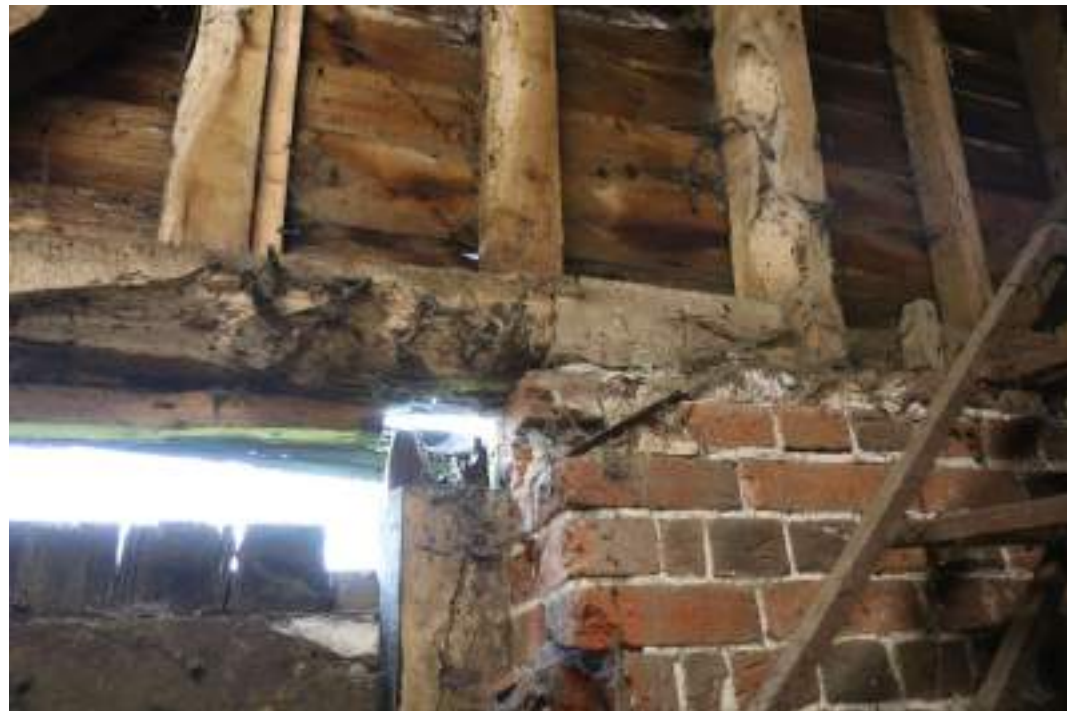
MGWF24_Phograph_136 Interior detail shot of side-halved scarf-joint on sill-beam above doorway in bay 3 of threshing barn. Photograph taken facing east.
