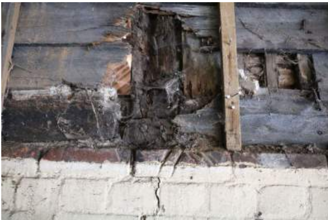
MGWF24_PhotoGraph_163 Interior detail shot of scarf-joint in northern sill-beam of lean-to 3. Photograph taken facing north.
