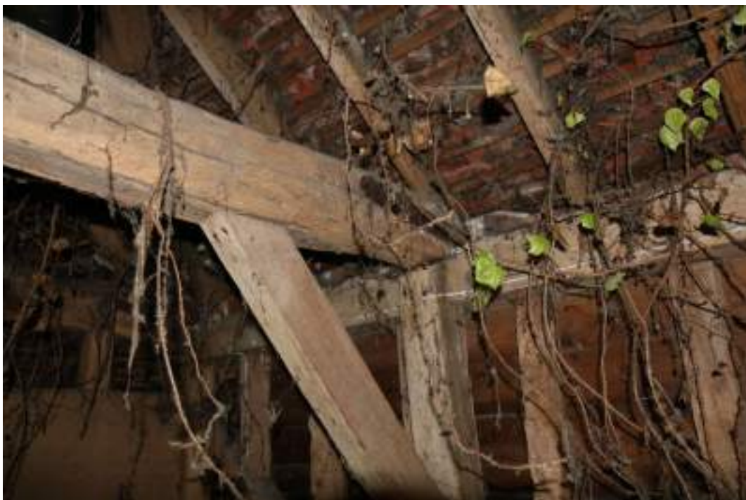
MGWF24_Phograph_119 Interior detail shot of inserted tie-beam and intermediate-post in bay 1 of threshing barn. Photograph taken facing north-east.
