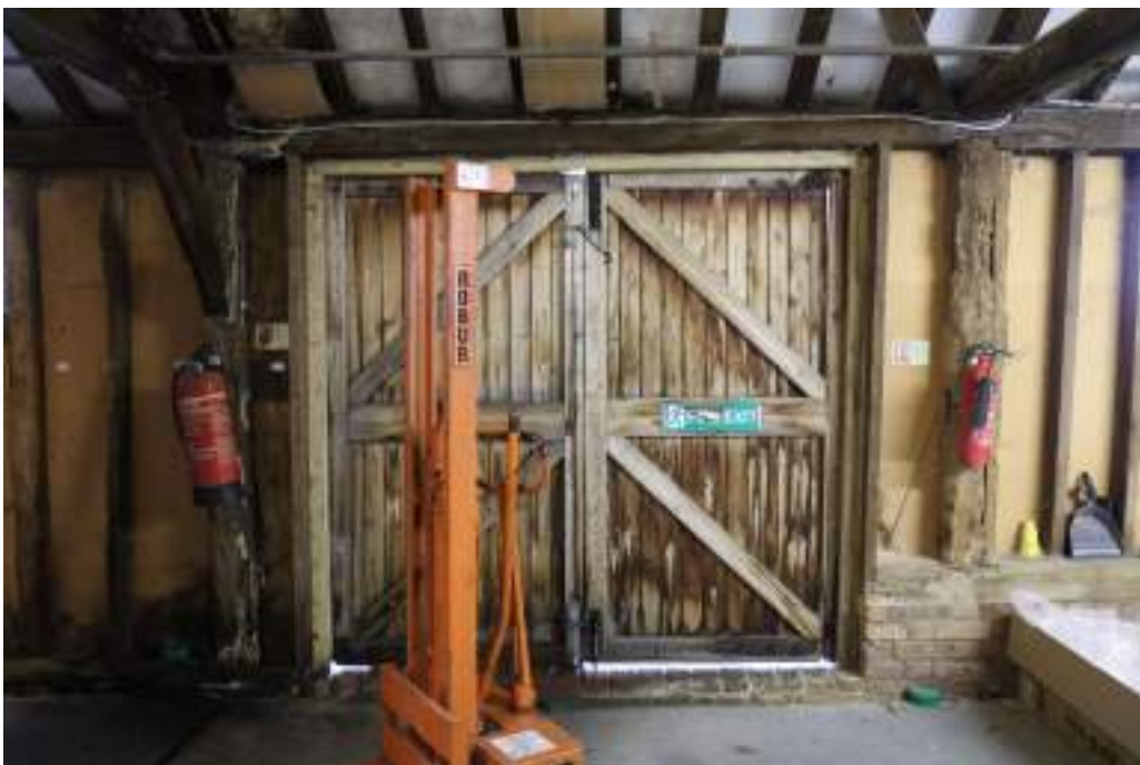
Photograph 44 Detail of doors in bay 3 of small barn, also showing the differing plinth heights either side. Photograph taken facing south.
