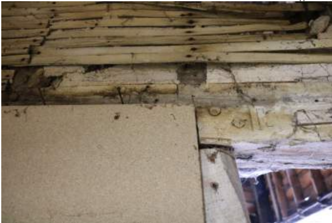
MGWF24_PhotoGraph_113 Interior detail shot of scarf-joint and carpenter's mark on sill-beam in lean-to 1. Photograph taken facing south.
