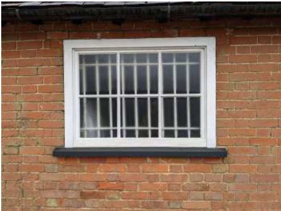
MGWF24_PhotoGraph_199 Detail shot of window on northern elevation of brick building. Photograph taken facing south.
