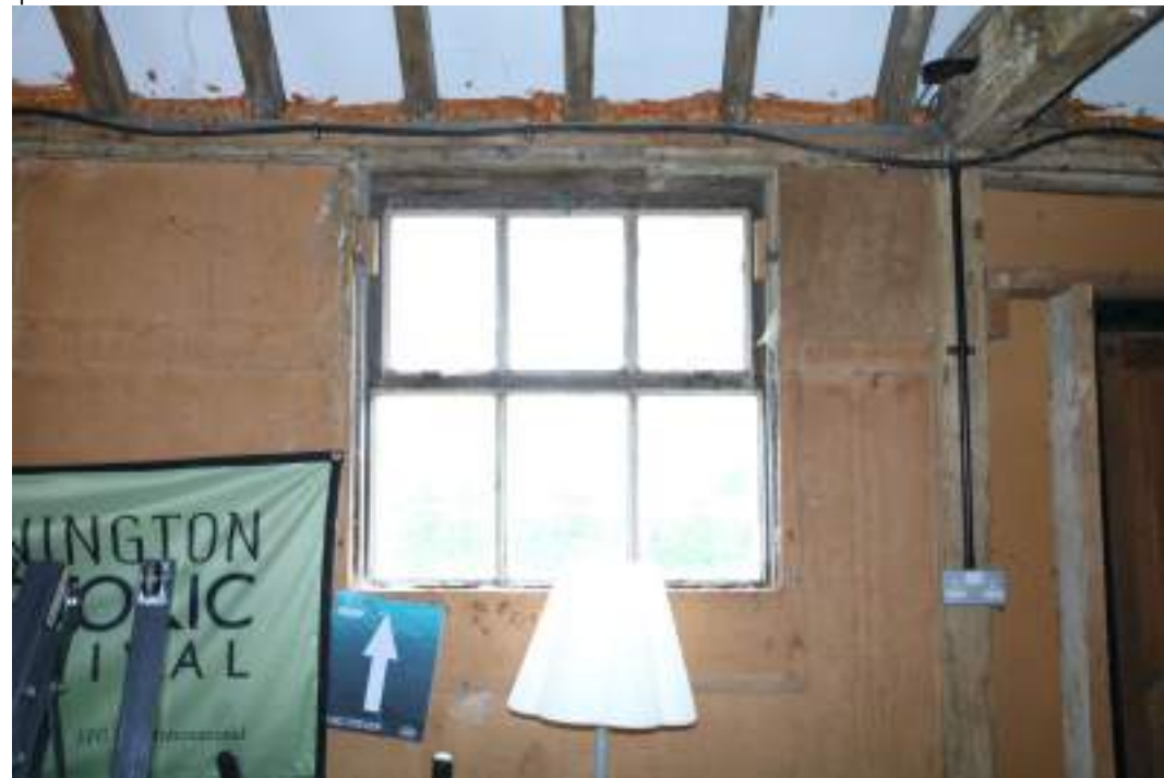
MGWF24_PhotoGraph_018 Interior shot of inserted metal framed window in cowshed, bay 4. Photograph taken facing west.
