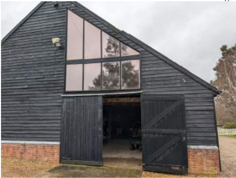
MGWF24_PhotoGraph_197 Detail of windows and door on southern elevation of cowshed. Photograph taken facing north.
