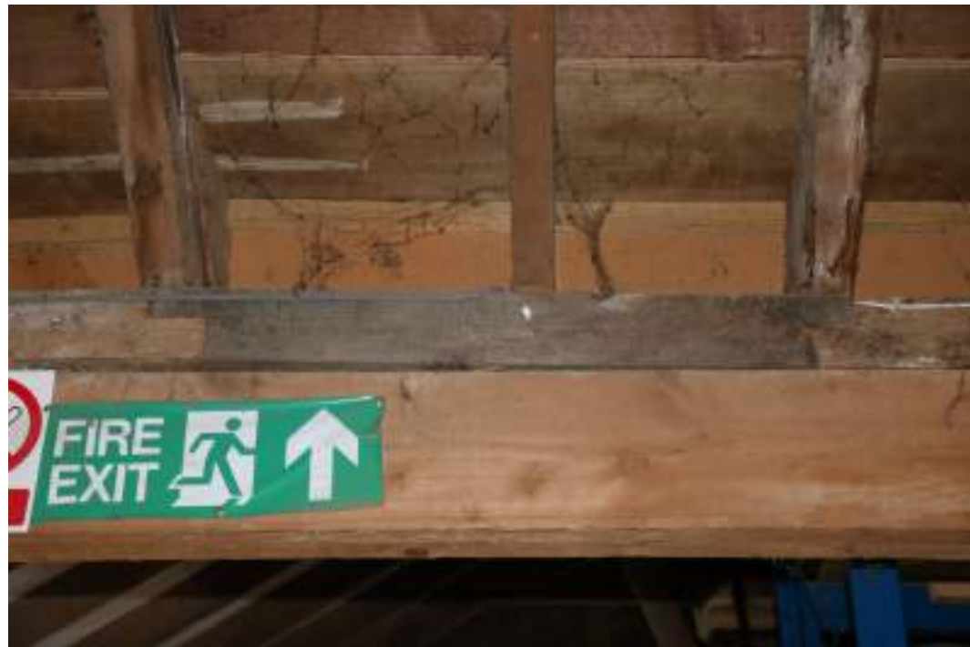
MGWF24_PhotoGraph_024 Interior detail shot of replacement timber and scarf-joints of wall-plate in cowshed, bay 7. Photograph taken facing west.
