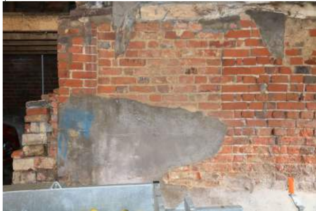
MGWF24_PhotoGraph_158 Interior detail shot of blocked doorway in midstrey of threshing barn. Photograph taken facing south.
