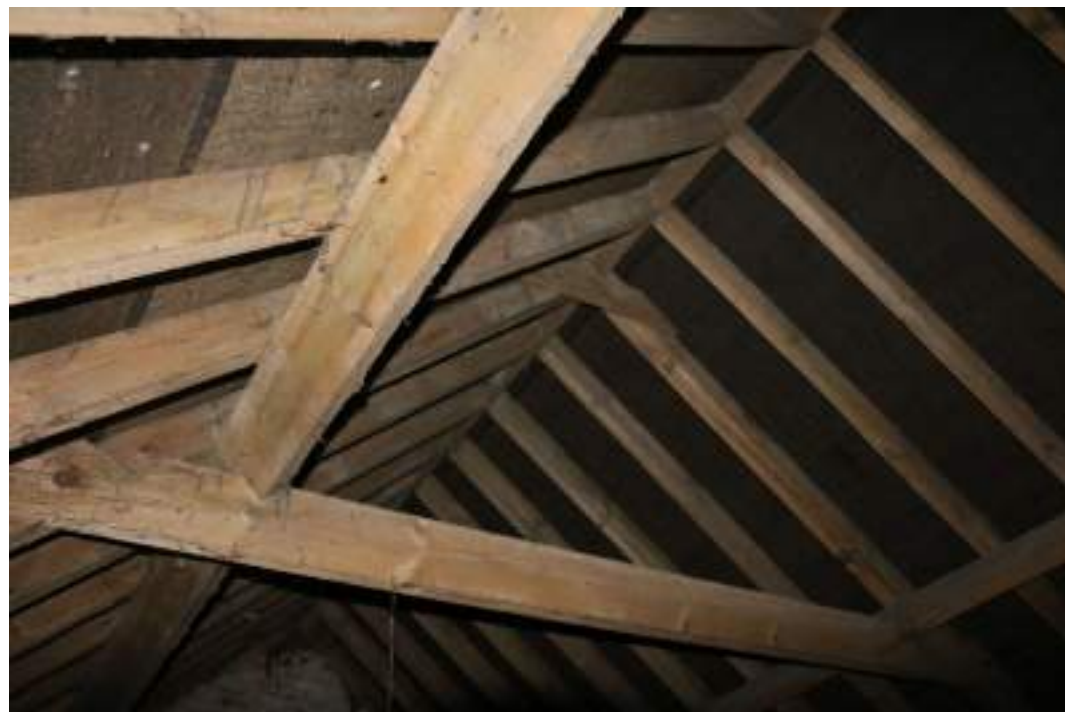
MGWF24_PhotoGraph_032 Interior detail shot of roof construction in brick building. Photograph taken facing north-west.
