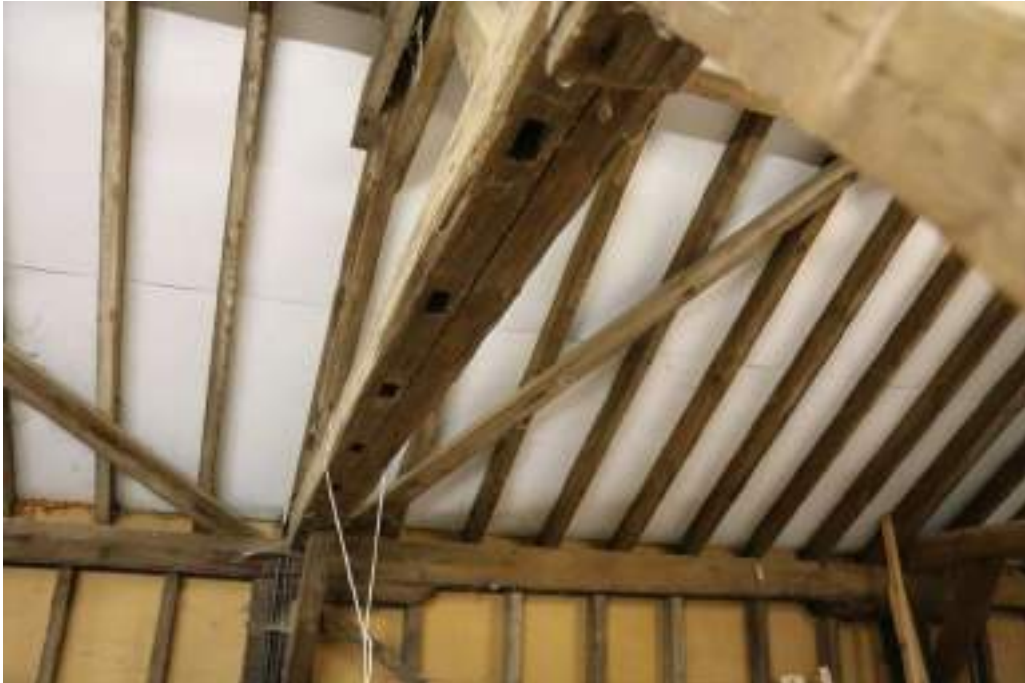
Photograph 43 Detail of reused tie-beam between bays 2 and 3 of small barn. Photograph taken facing north-east.
