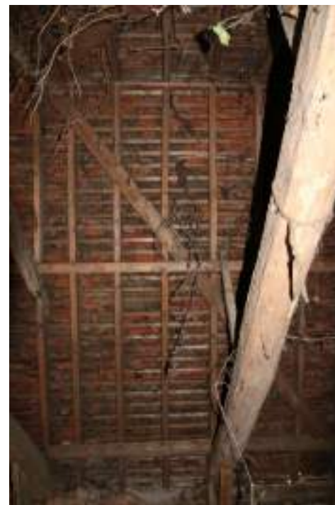
MGWF24_PhotoGraph_116 Interior detail shot of roof construction in bay 1 threshing barn. Photograph taken facing west.
