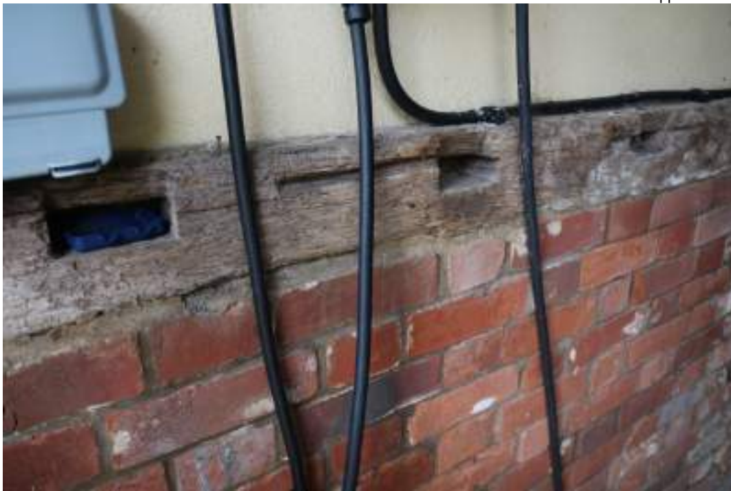
MGWF24_PhotoGraph_097 Interior detail shot of reused timber sill-beam in carport. Photograph taken facing north-east.
