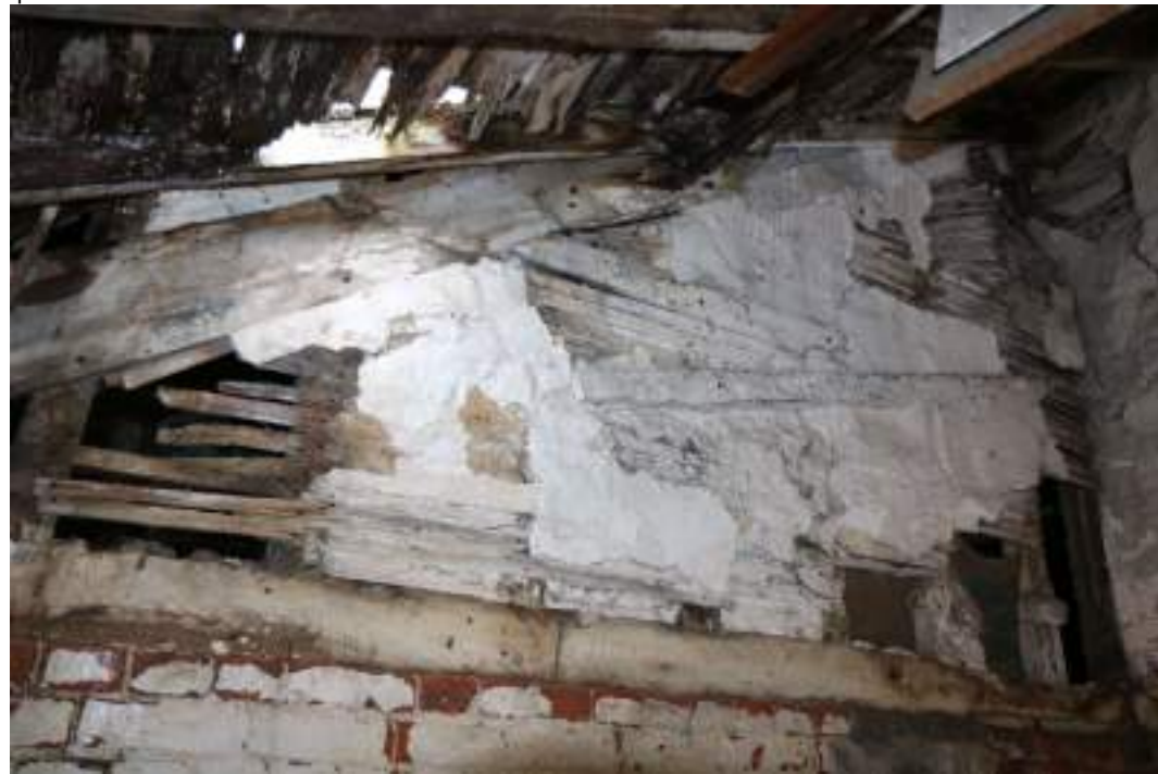
MGWF24_PhotoGraph_078 Interior detail shot of laths and plaster wall in lean-to 2. Photograph taken facing north-east.
