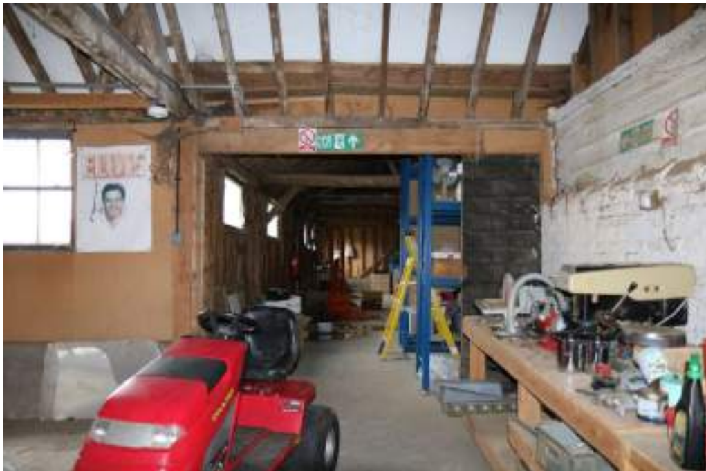
Photograph 35 Detail of opening between cowshed and small barn. Photograph taken facing west.
