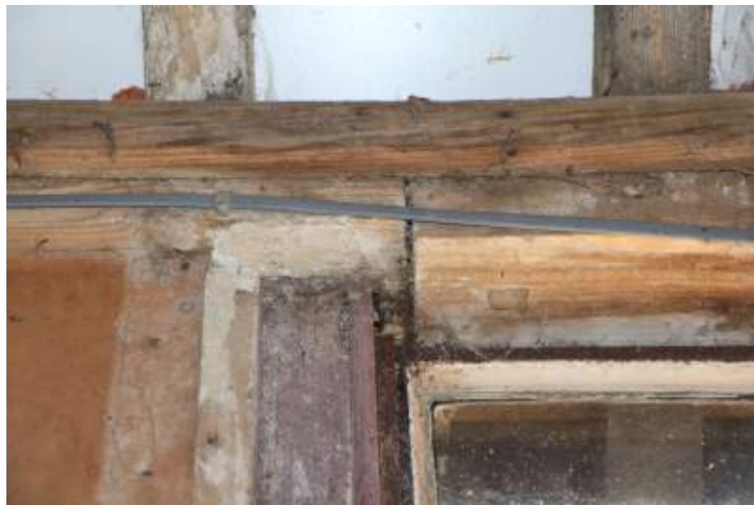
MGWF24_PhotoGraph_012 Interior shot of simple scarf-joint in wall-plate of cowshed, bay 3. Photograph taken facing east.
