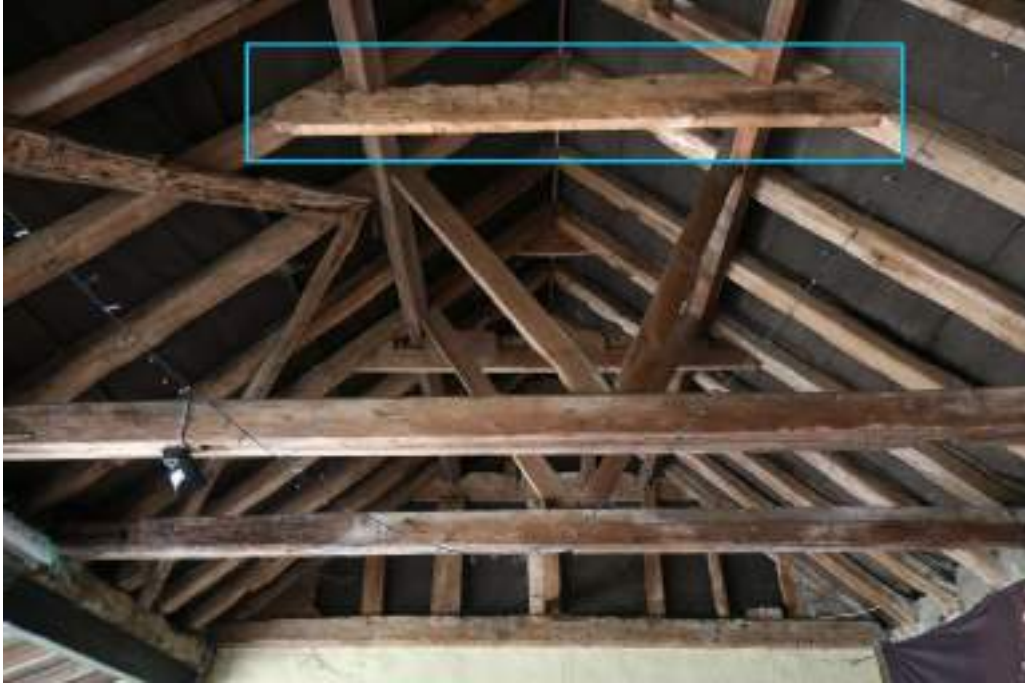
Photograph 23 Detail of carport roof construction. A collar with lap-dovetailed joints highlighted in blue. Photograph taken facing north.
