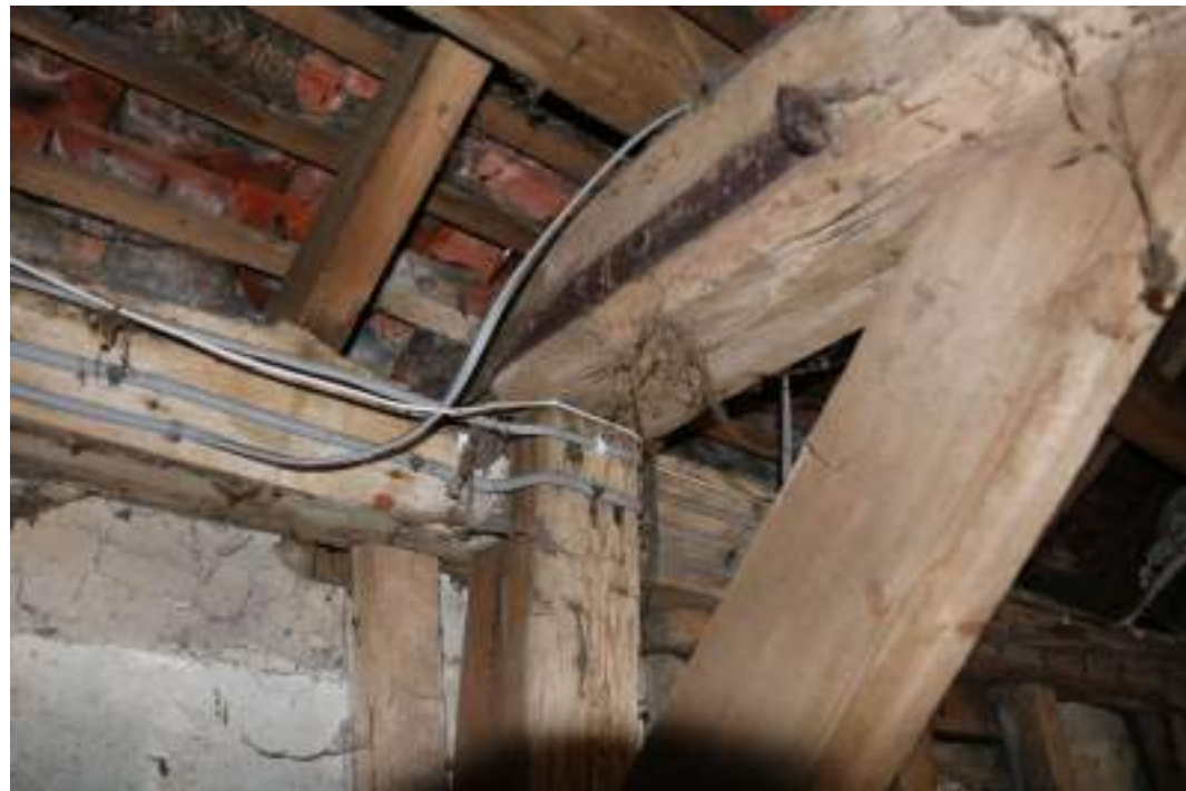
MGWF24_PhotoGraph_148 Interior detail shot of iron strap on inserted tie-beam and intermediate post in bay 4 of threshing barn. Photograph taken facing north-west.
