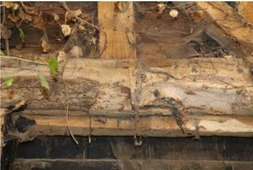
MGWF24_Phograph_135 Interior detail shot of side-halved and bridled scarf-joint on sill-beam above doorway in bay 3 of threshing barn. Photograph taken facing east.
