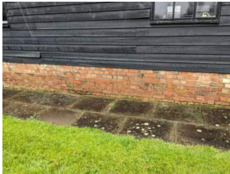
MGWF24_PhotoGraph_192 Detail shot of brick plinth on western elevation of cowshed. Photograph taken facing east.
