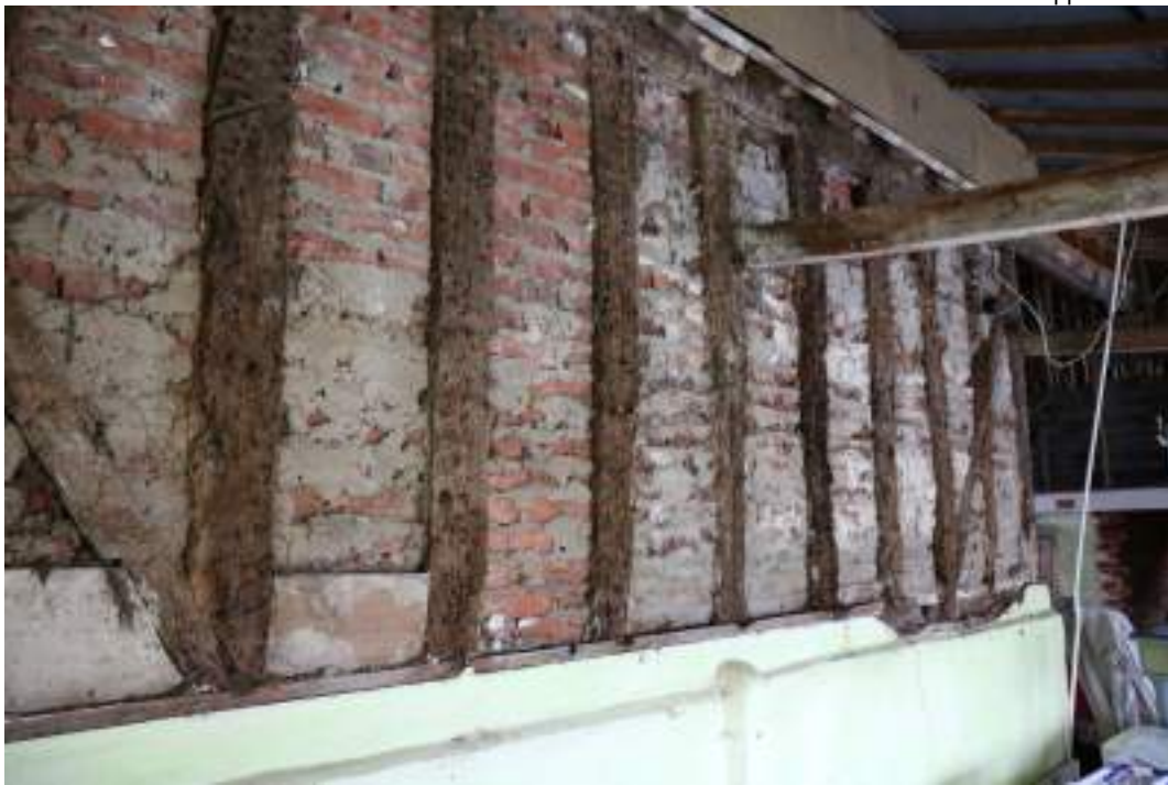
MGWF24_PhotoGraph_161 Interior detail shot of wall construction lean-to 3. Photograph taken facing north-west.
