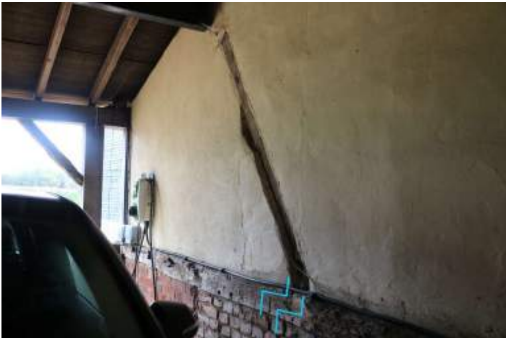
Photograph 24 Detail of exposed wind-brace in carport. Wall-plate scarf-joint highlighted in blue. Photograph taken facing north-west.
