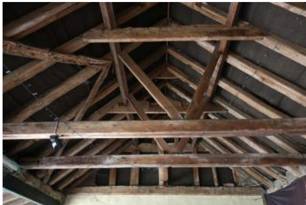
MGWF24_PhotoGraph_092 Interior shot of roof structure of carport. Photograph taken facing north.
