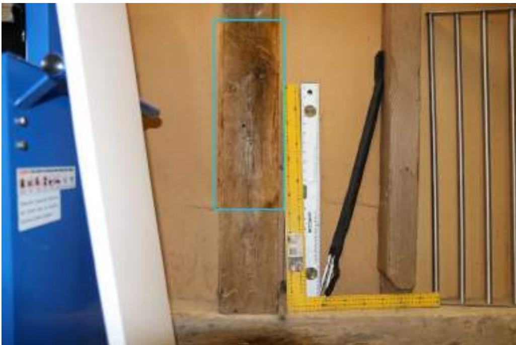
Photograph 40 Detail of Baltic timber mark on intermediate-post of bay 1 of small barn. Photograph taken facing west.
