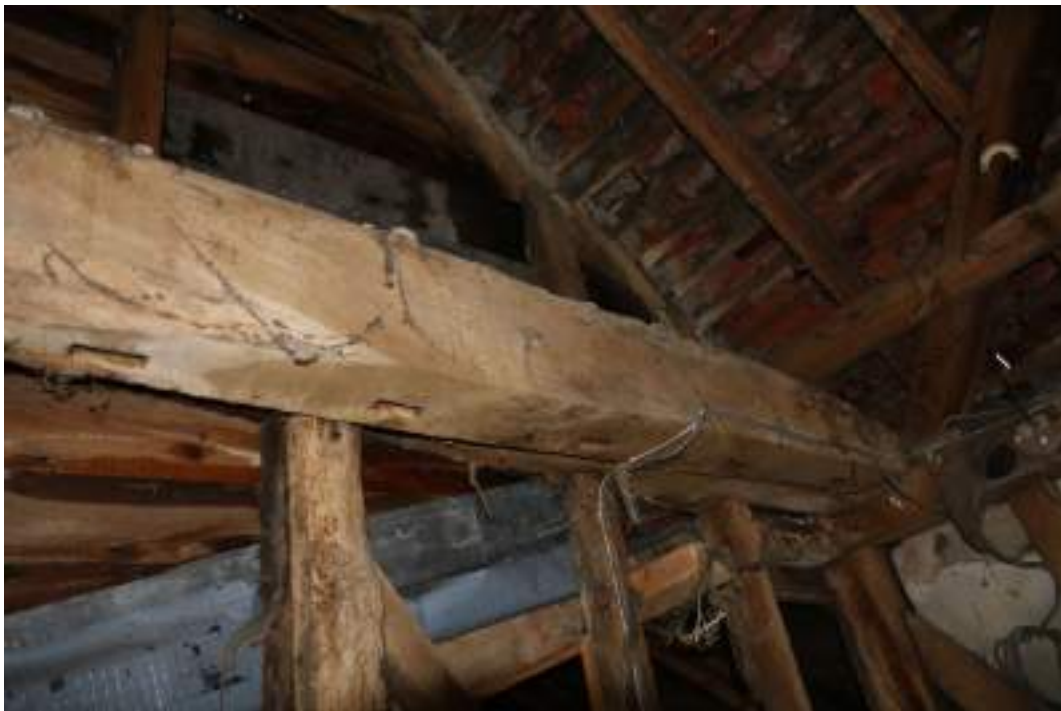
MGWF24_PhotoGraph_147 Interior detail shot of reused timber tie-beam in bay 4 of threshing barn. Photograph taken facing south-west.
