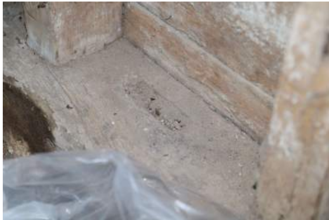
MGWF24_PhotoGraph_072 Interior detail shot of reused timber sill-beam in the small barn, bay 5. Photograph taken facing north-east.
