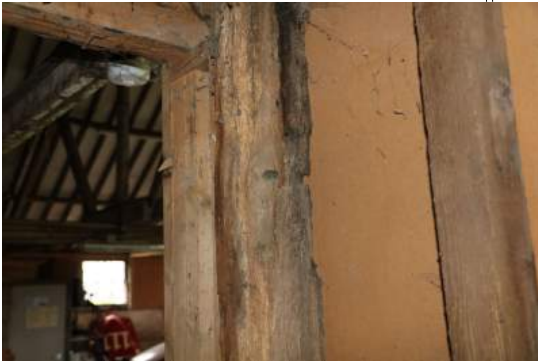
MGWF24_PhotoGraph_069 Interior detail shot of reused timber corner-post of small barn, bay 5. Photograph taken facing south-east.
