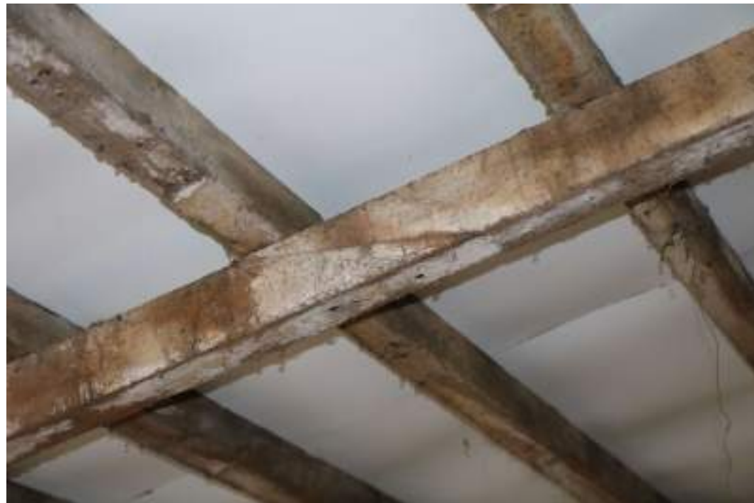
MGWF24_PhotoGraph_016 Interior detail shot of splayed scarf-joint in lower purlin of cowshed, bay 4. Photograph taken facing south-west.
