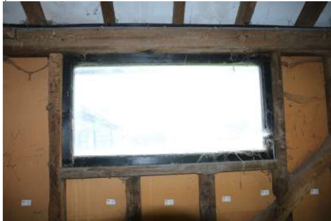
MGWF24_PhotoGraph_070 Interior shot of roof construction in barn, bay 5. Photograph taken facing south.
