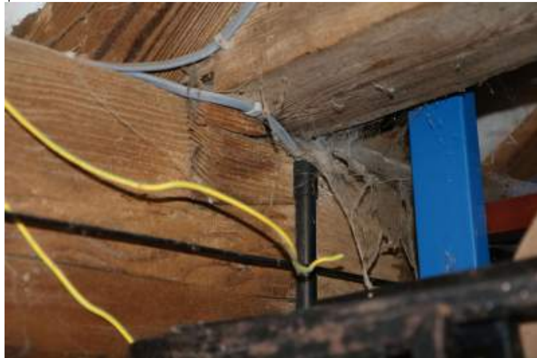
MGWF24_Phograph_062 Interior detail shot of scarf-joint on wall-plate under tie-beam between bays 4 and 5, small barn. Photograph taken facing north-east.
