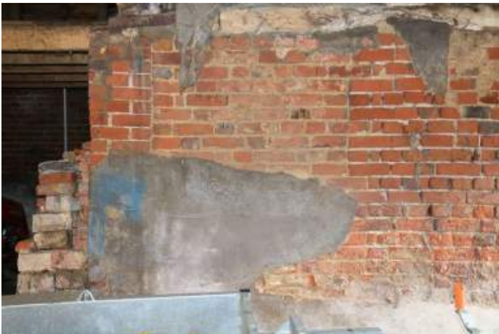
Photograph 16 Detail of blocked doorway in midstrey of threshing barn. Photograph taken facing south.
