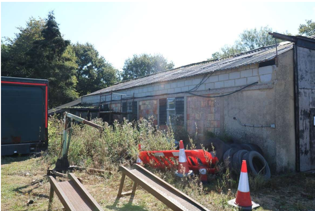
Photograph 12 Northern elevation of building 5, with detail of the raised roof. Photograph taken facing south-east.
