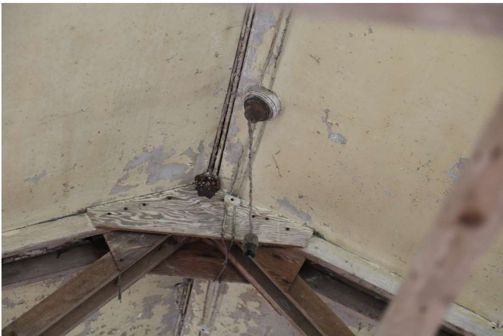
Photograph 19 Detail of light fitting in building 7. Photograph taken facing north-west.
