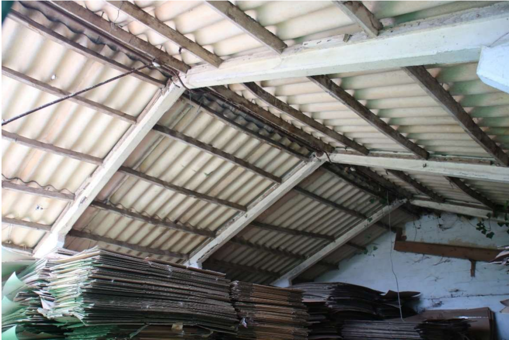
Photograph 2 Roof structure of a MoWP standard hut (building 18). Photograph taken facing north-east.
