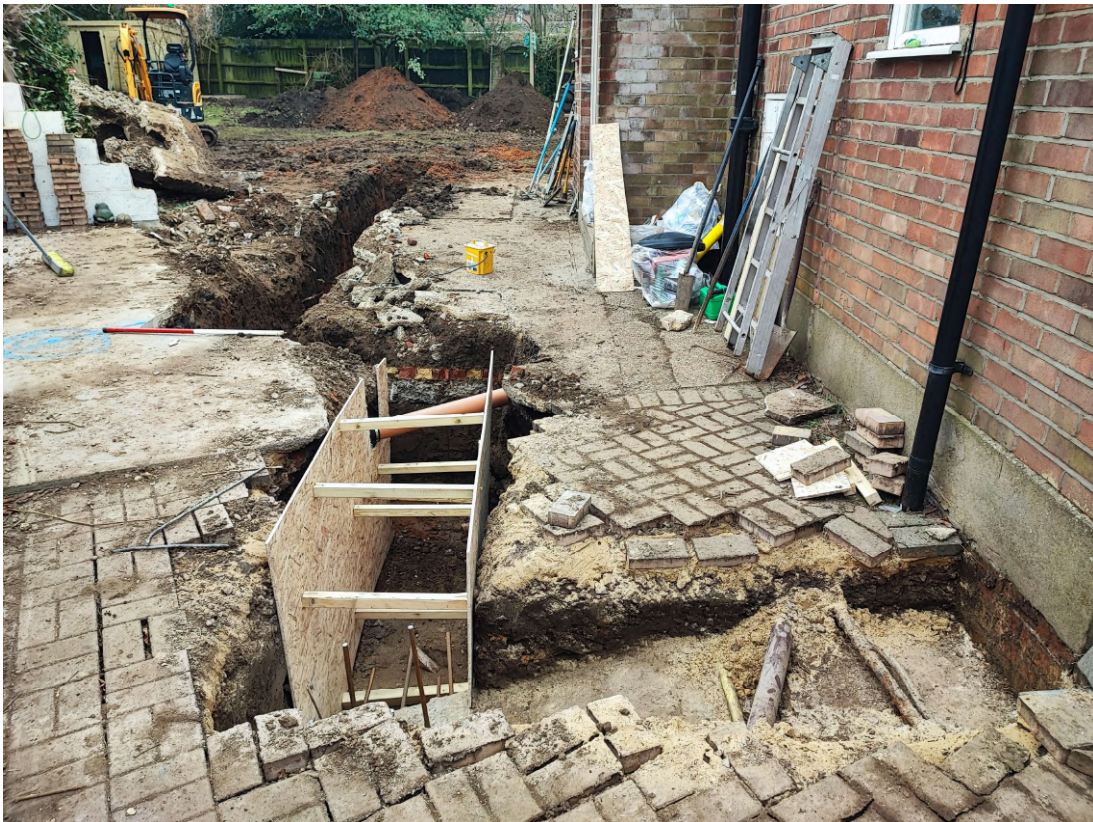
Photograph 3 The northern half of the foundation trench showing concrete slab/block F2 in foreground, looking south-south-west.
