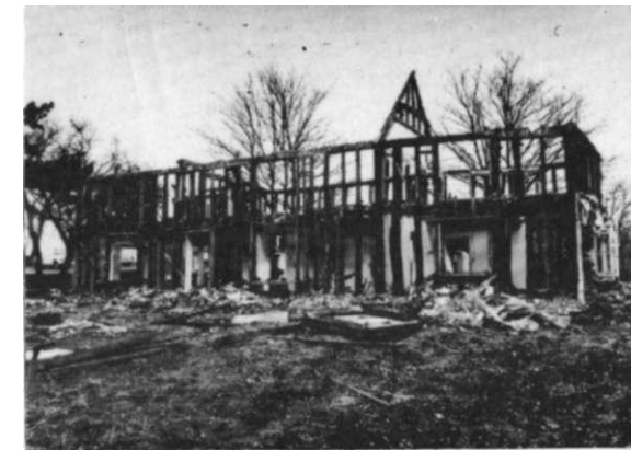
The timber framing of Poplarhall Farm showing after removal of modern cladding.
