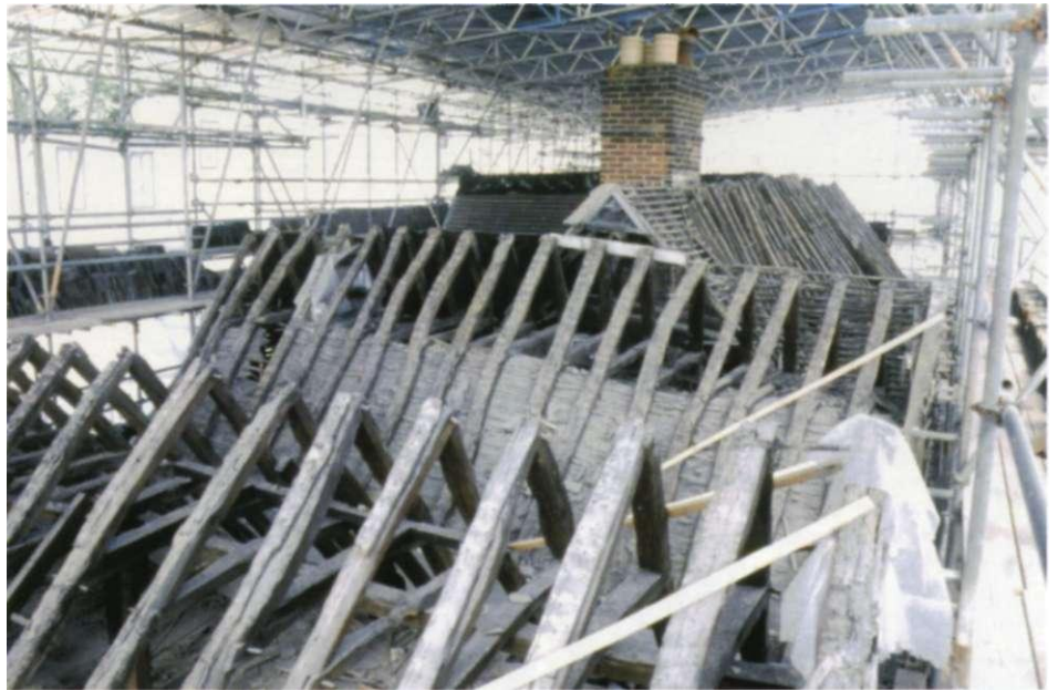
A remarkable bird's-eye view of the medieval roofs, stripped of tiles, from the dizzy heights of the scaffold.
